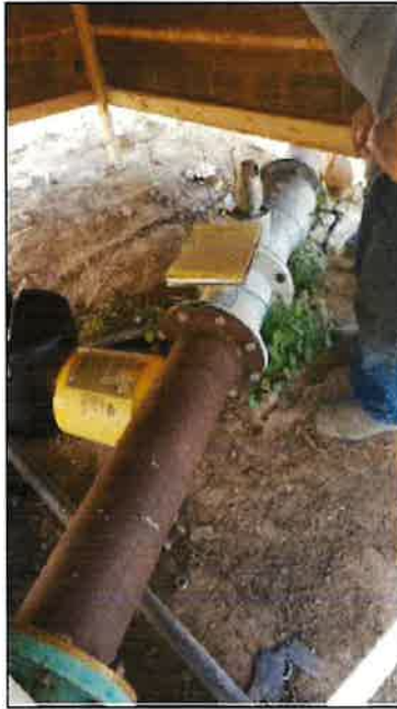
Figure 3: Discharge pipe of Well 1 showing flowmeter location.
