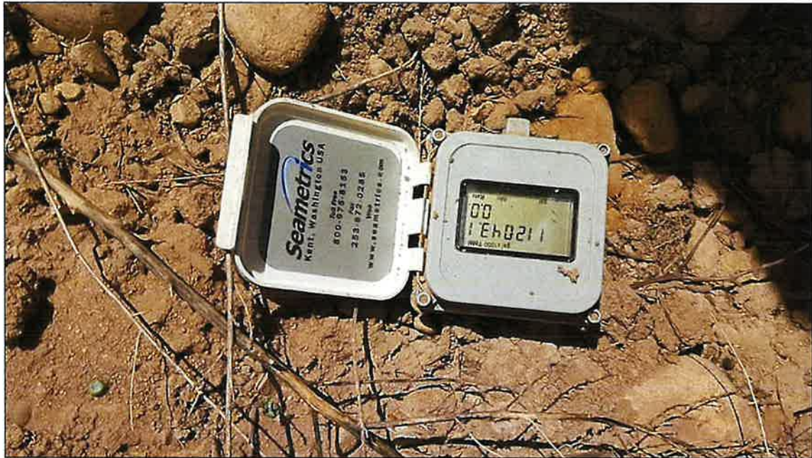
Figure 5: Flowmeter installed north of Kuna-Mora road on pipeline serving 63-33401 place of use.
