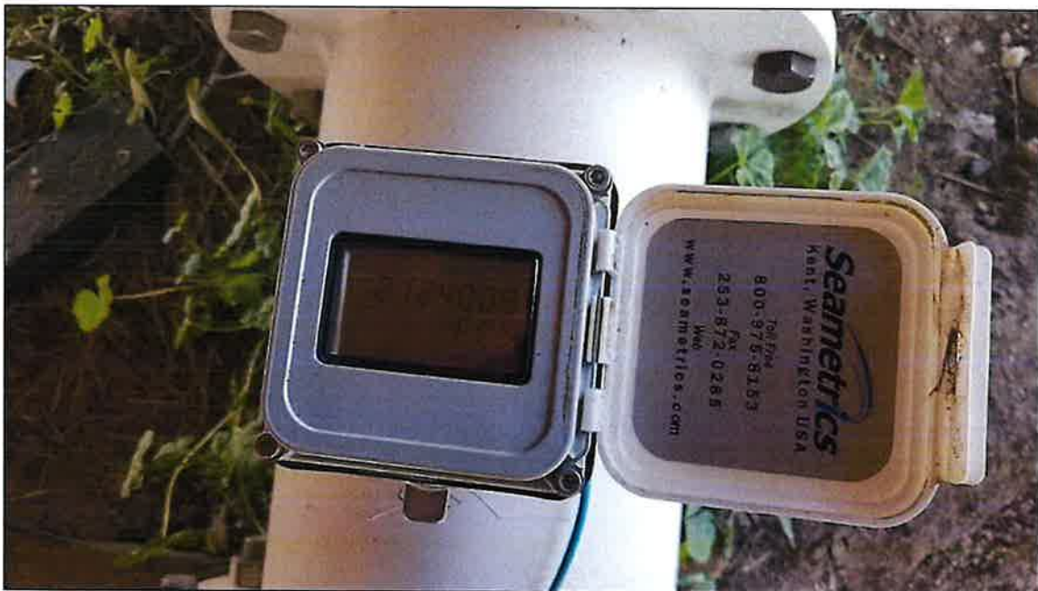
Figure 2: Flowmeter installed on Well 1.
