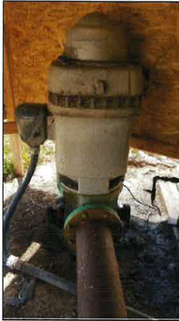
Figure 1: Well 1 75-hp vertical turbine.
