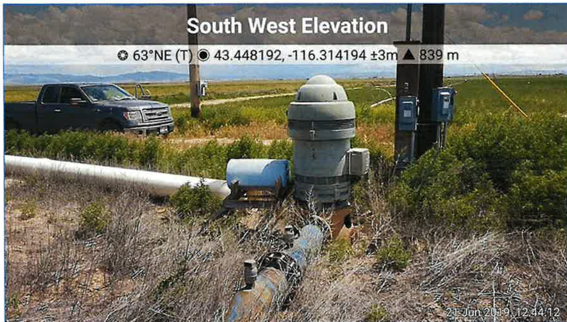
Figure 11: Well 4 equipped with 150 hp motor and vertical turbine pump.
