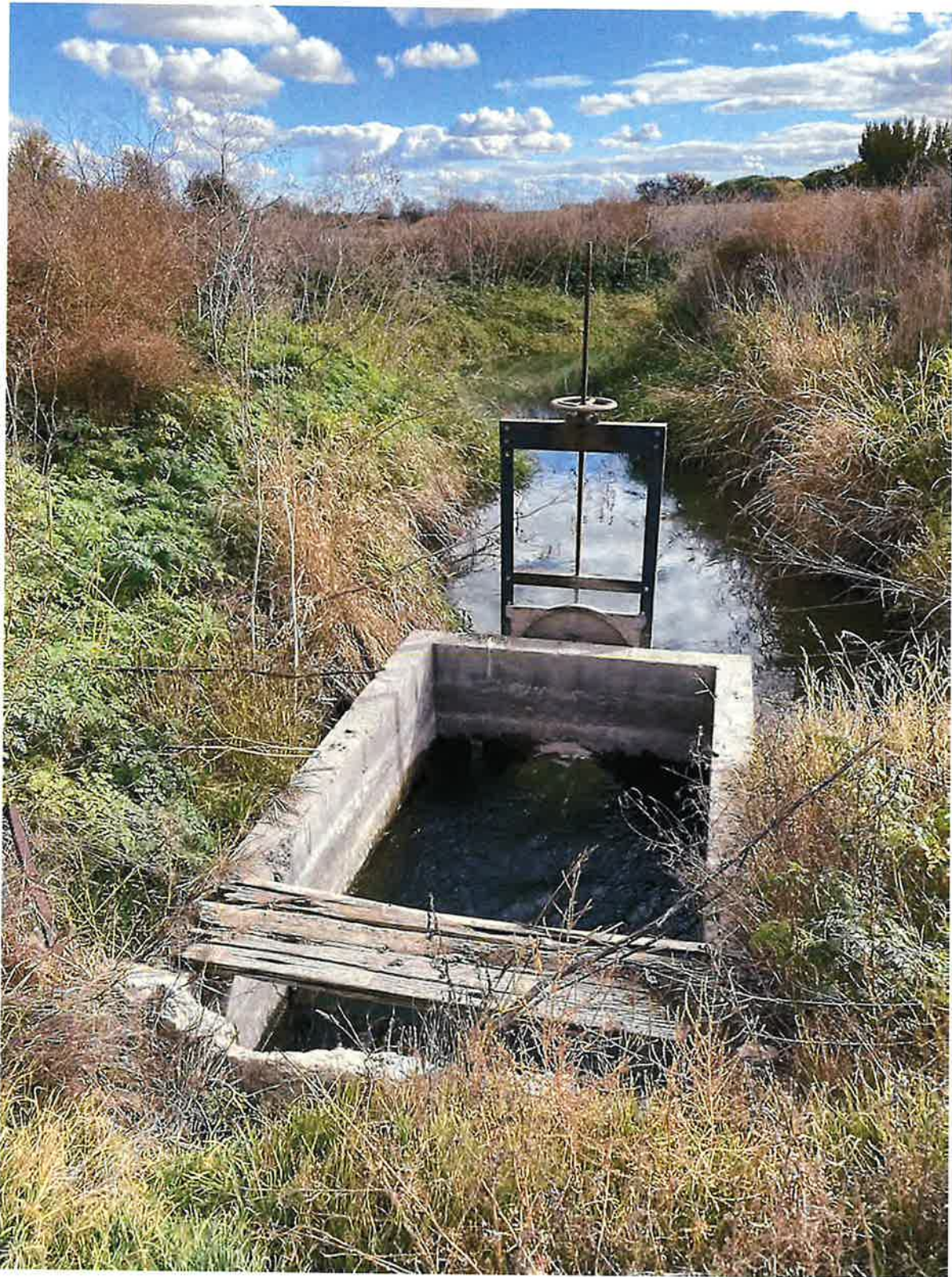
Lockable headgate at point of diversion.
