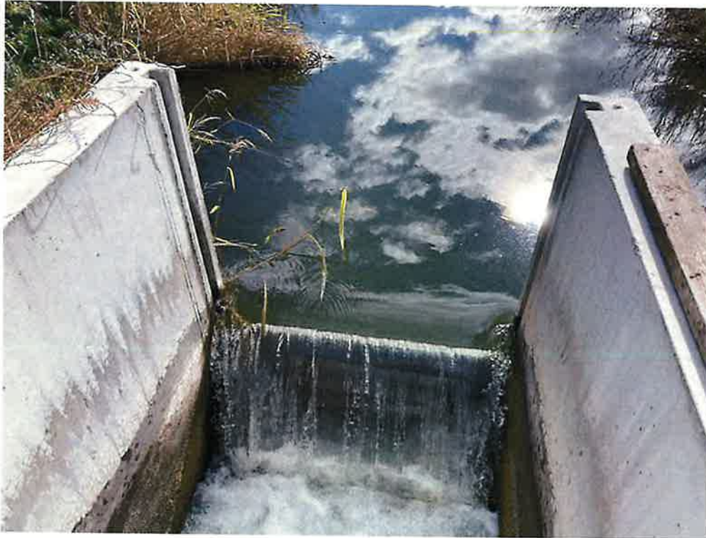
Check structure at head of North Ditch at bifurcation of Upper Haas Ditch. Boards function as a 4-foot suppressed weir
