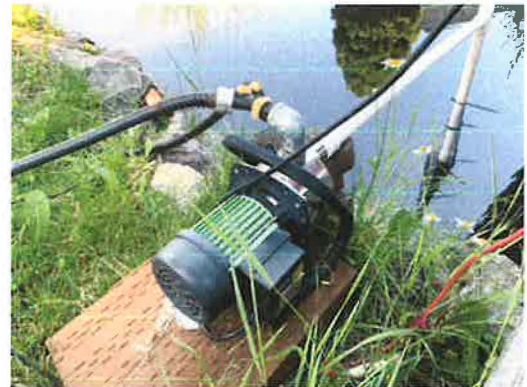
The electric pump is a third HP. A connector attaches 2 hoses to the pump, which can be used separately, together, and at adjustable output levels.
