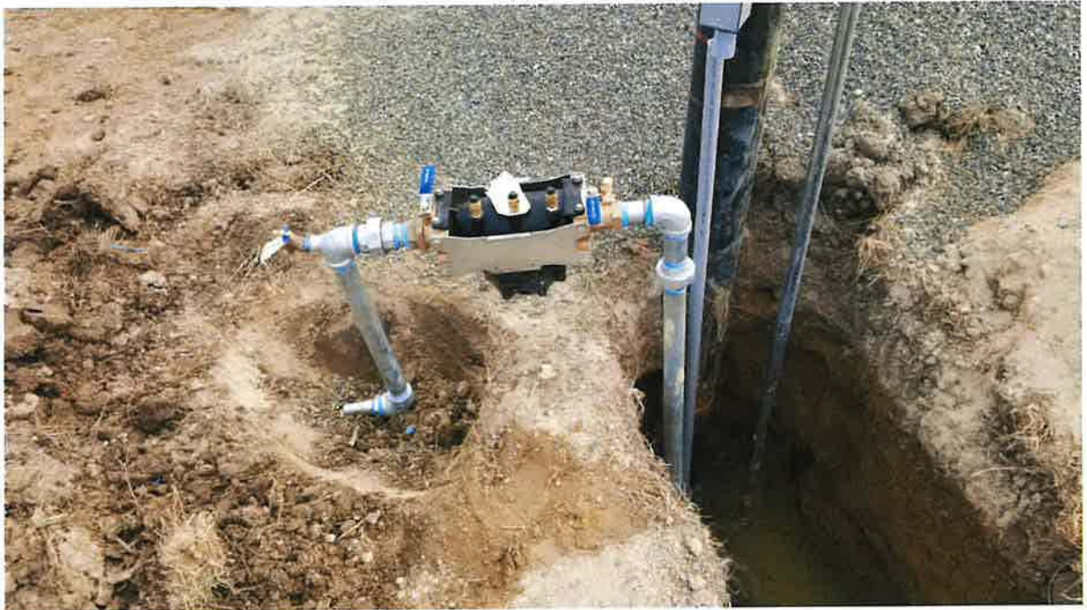
Figure 2 - Well and Sprinkler Manifold
