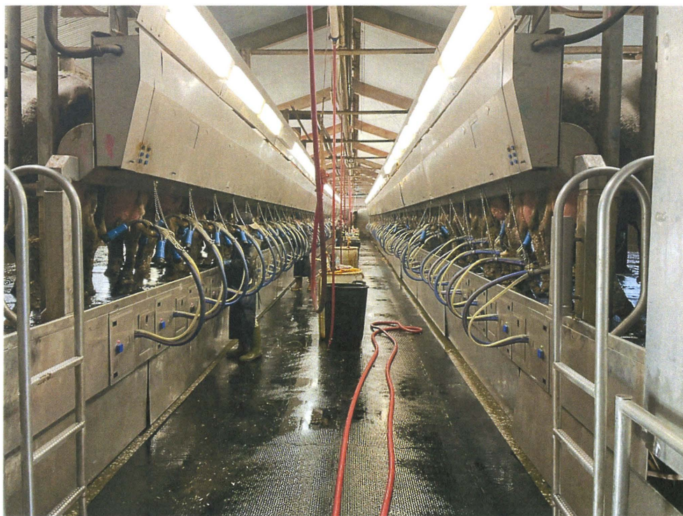
Figure 22 Milking bay featuring nine, 1" hoses with a Gilmour brand rear control cleaning nozzle.
