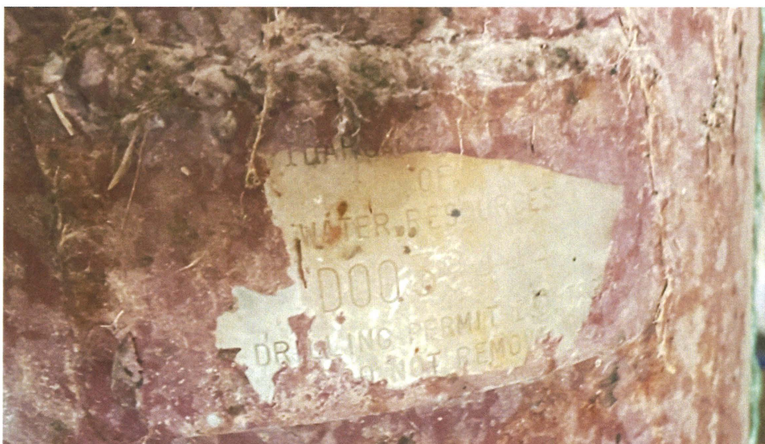
Figure 14 Tag to well D0039444 for stockwater and commercial use.
