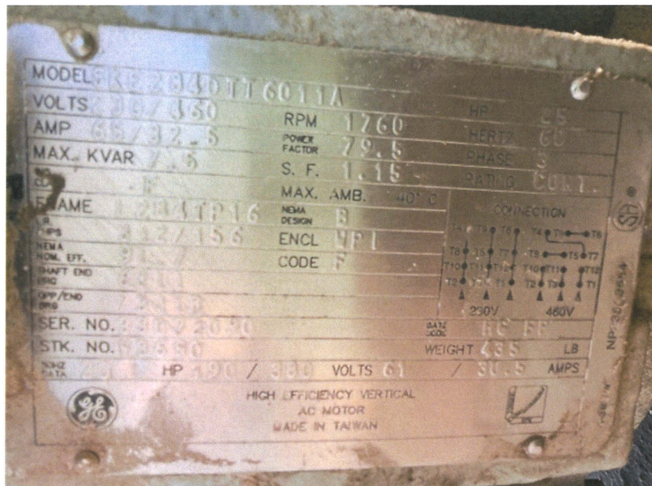
Figure 7 Pump tag for 25hp pump associated with storage pond.
