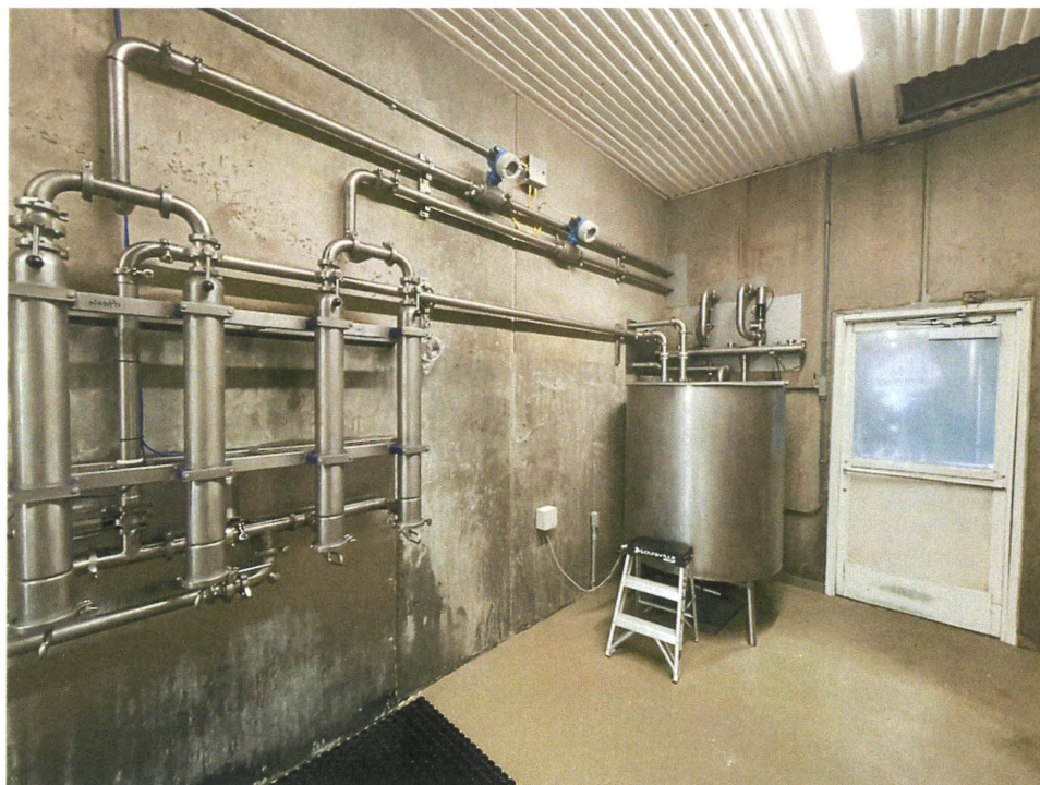
Figure 20 Clean-in-Place system and milk transfer lines.
