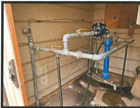
Photo 9 (above) - 1 1/4" Galvanized risers with flowmeter and pressure sensors.
