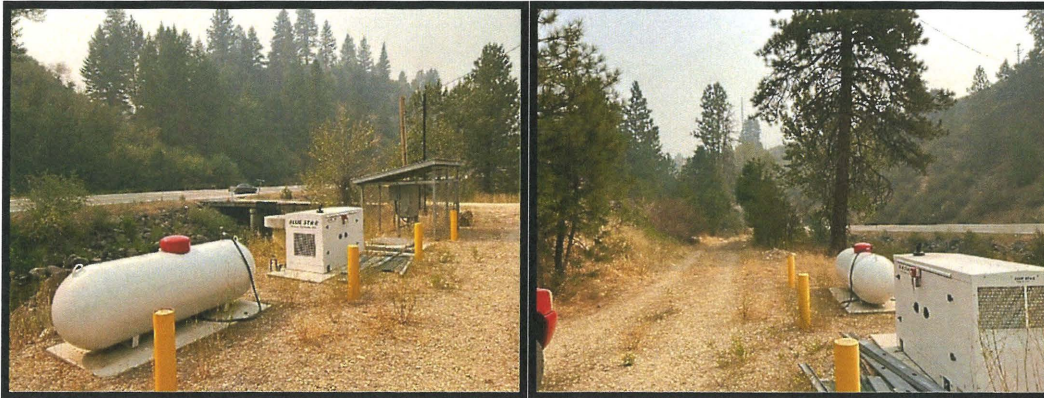
Photo 23 (Left)- Mores Creek surface water diversion from wet well (GPS Coords: N43°39.102' W115°58.839'. Photo 24 (Right)- The water main was bored in from the round vault to the water treatment plant just to the right of the cell tower visible on the ridgeline in the background.
