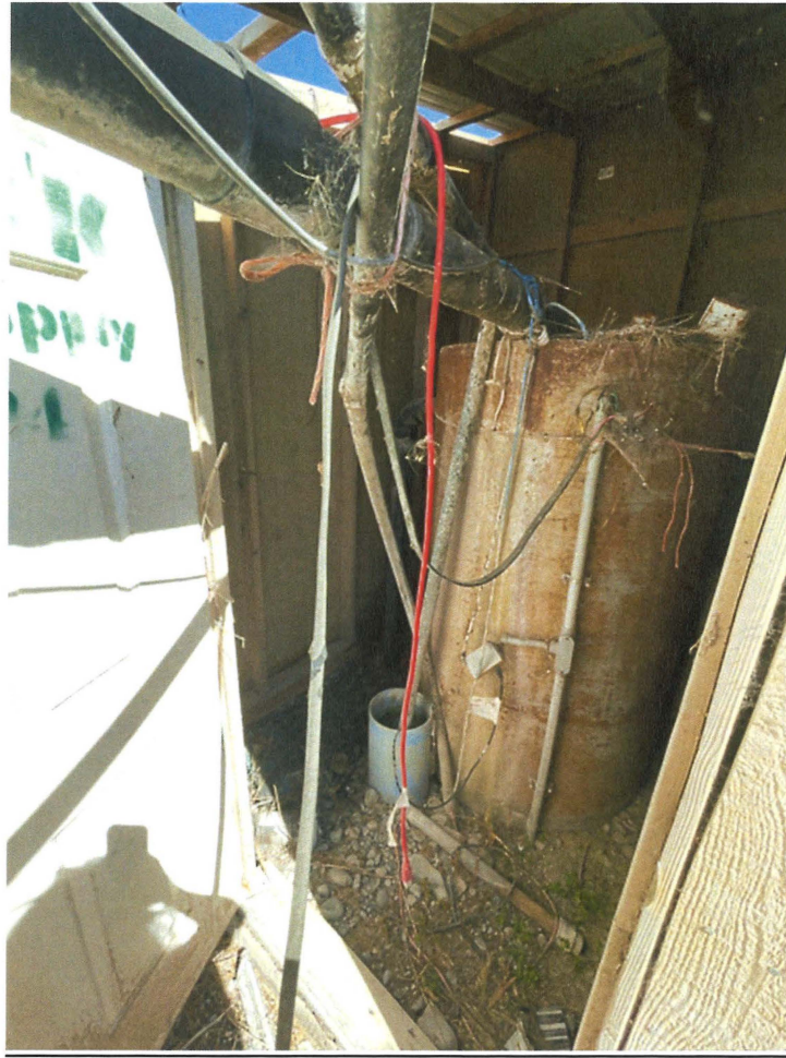
Figure 2 Point of diversion including power source for 5hp pump from spring and 1.25" pipe diverting water to storage tank.
