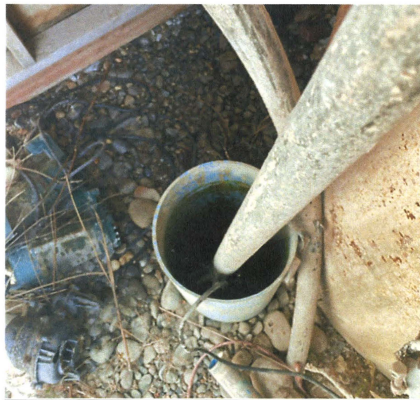
Figure 3, 1.25" pipe diverting water from 5hp pump upwards towards storage tank.
