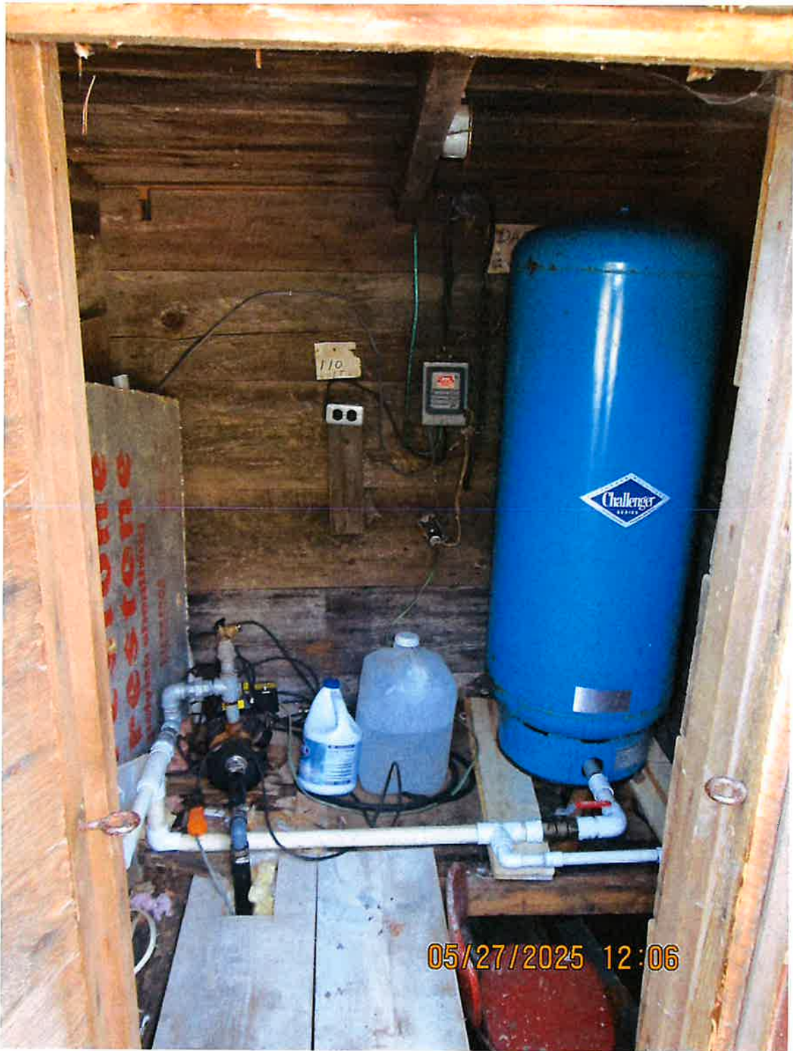
Image 3 – Pump house with pressure tank and ¾ HP jet pump
