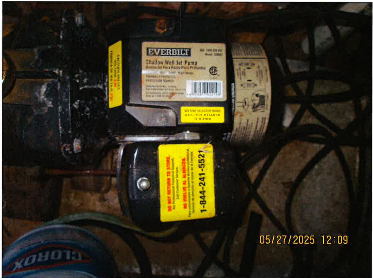
Image 4 – Well pump details
