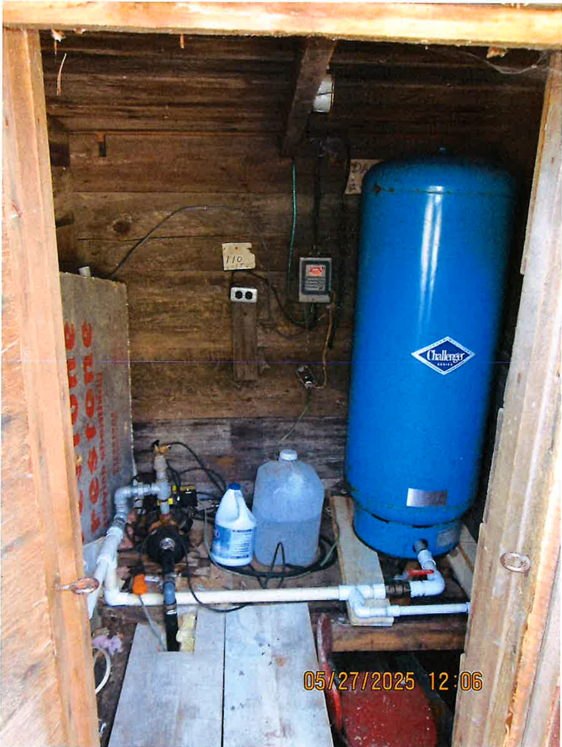
Image 3 – Pump house with pressure tank and ¼ HP jet pump
