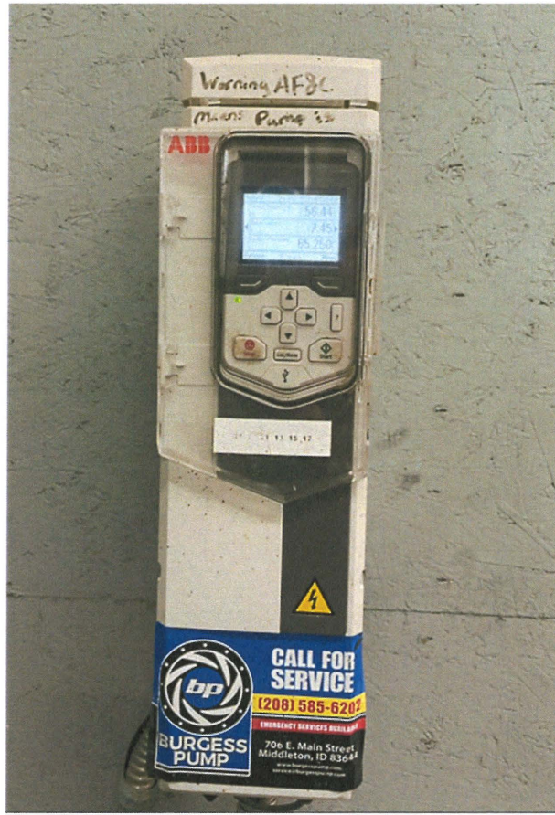
Figure 5 Front side of control panel for well 1.
