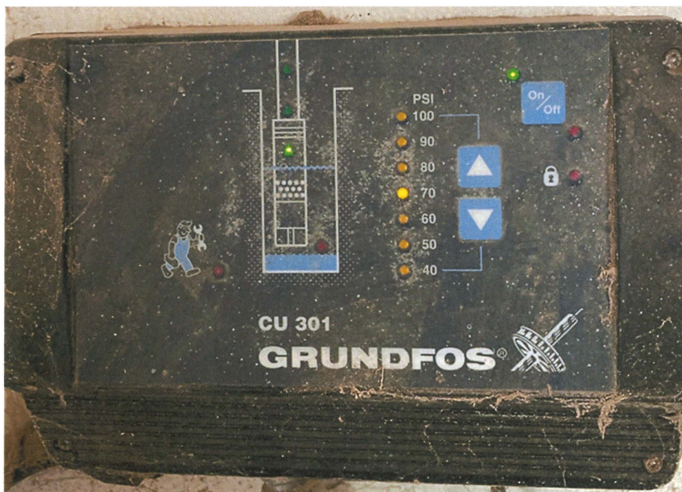
Figure 10 Grundfos CU 301 pressure control showing 70 psi for Well 3.
