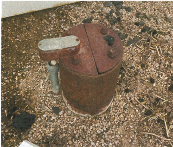
Figure 11 Well 4, no metal tag number found.
