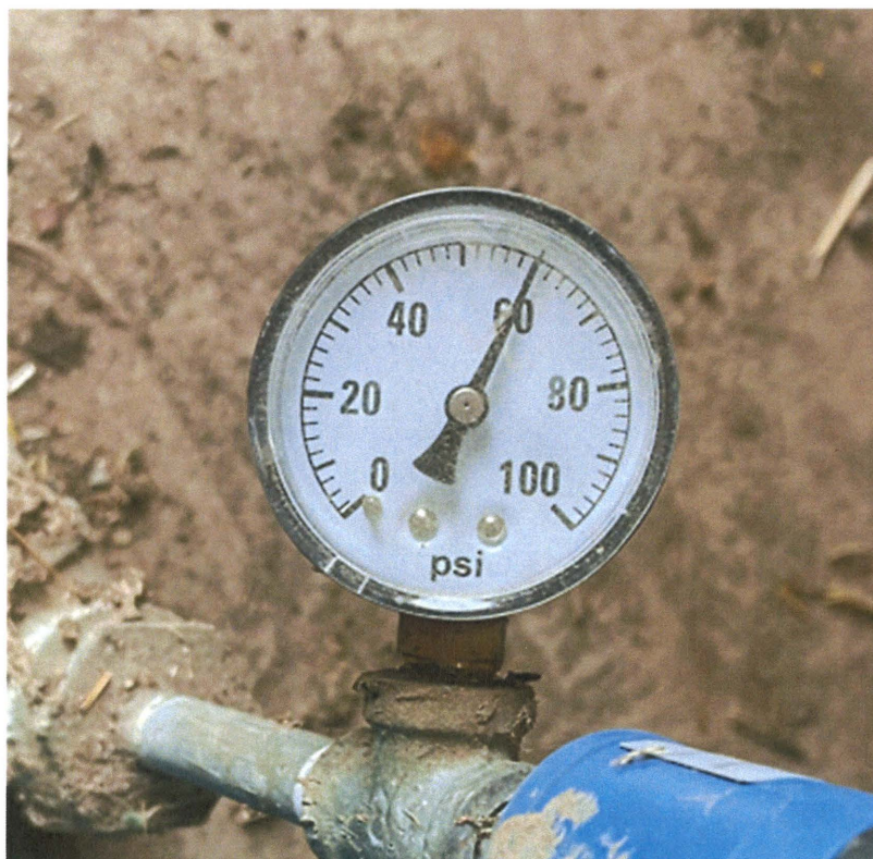
Figure 14 Pressure gage on Well 4, showing 60psi at the time of the field exam.
