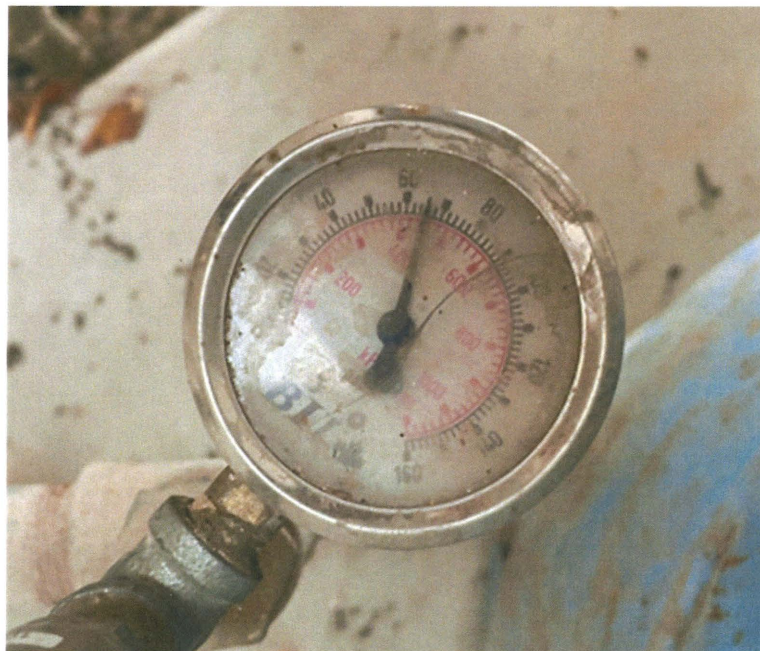
Figure 18 well 5 pressure gage showing 65 psi at the time of the field exam.
