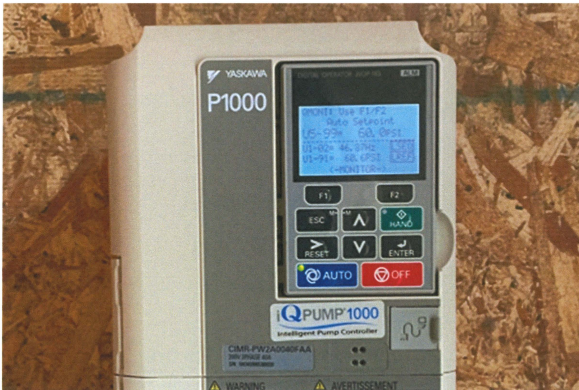
Figure 12 Yaskawa P1000 control panel showing 60 psi for Well 4.
