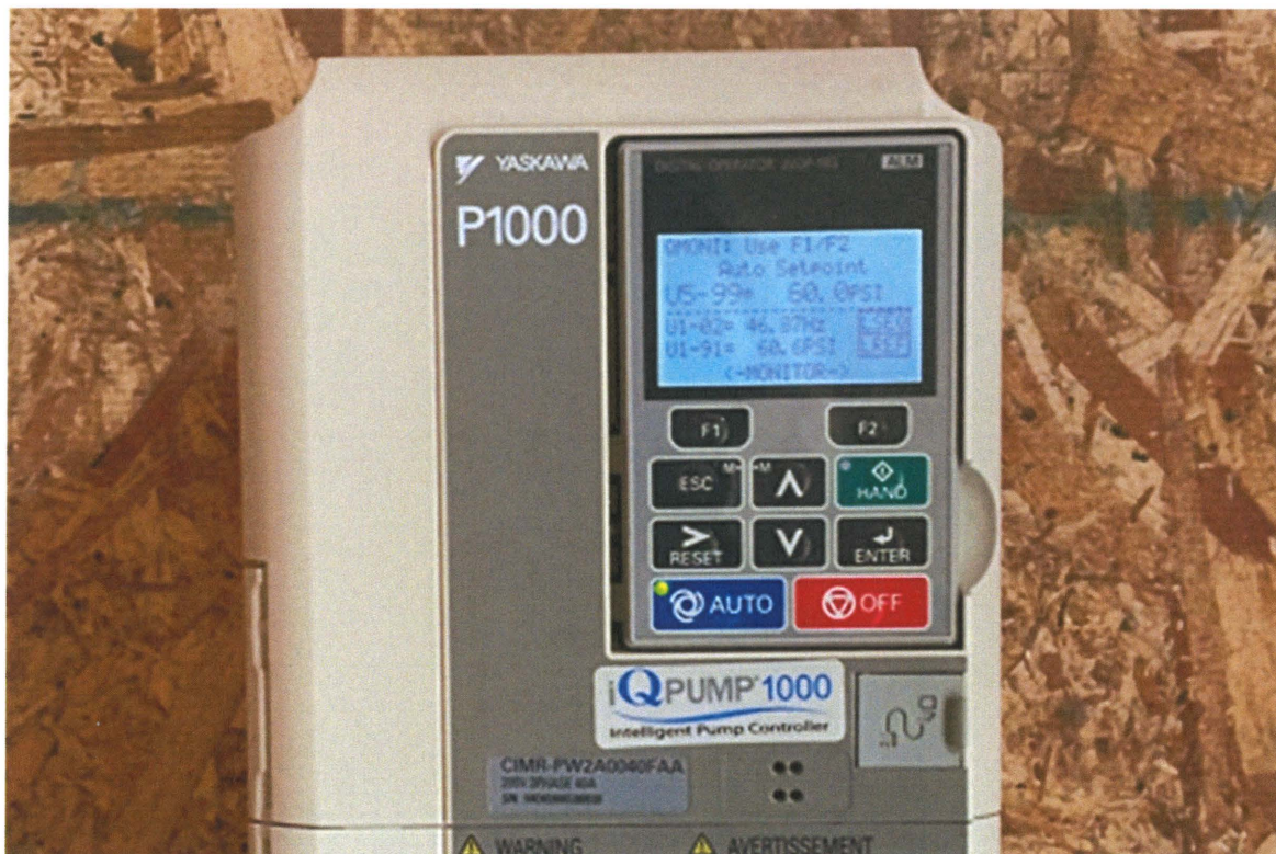
Figure 15 Yaskawa P1000 control panel showing 60 psi for Well 4.
