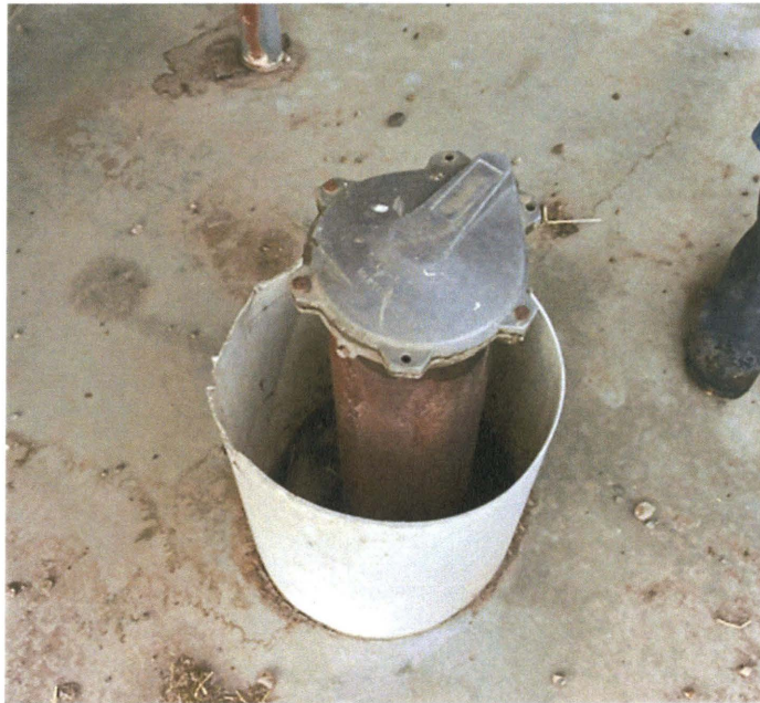
Figure 12 Well 3 with no identification tag.
