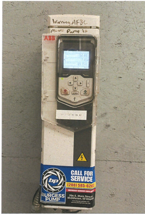
Figure 6 Control panel for Well 1.
