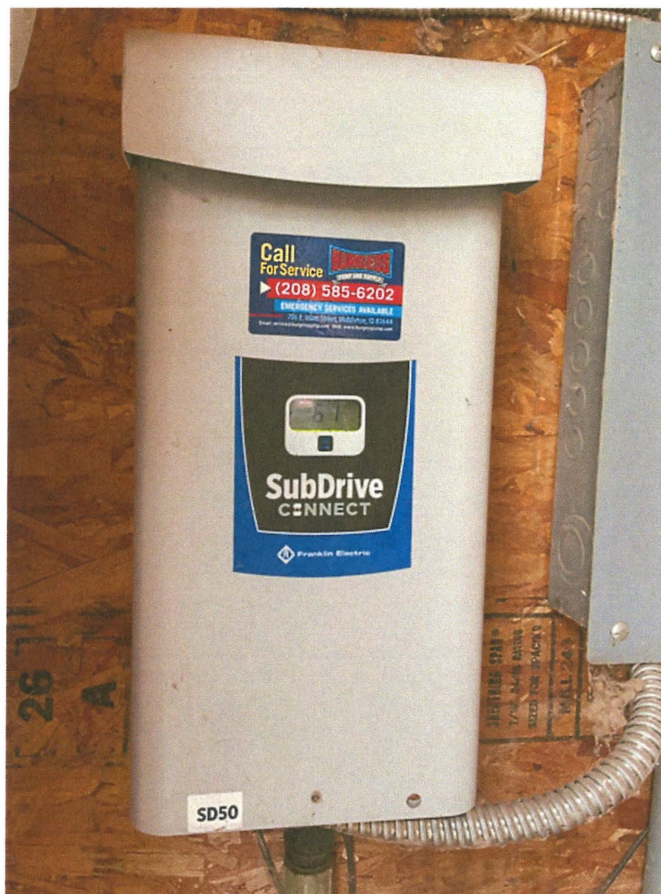
Figure 10 Franklin Electric SD50 Subdrive Connect control panel showing 61PSI for well D0031467.
