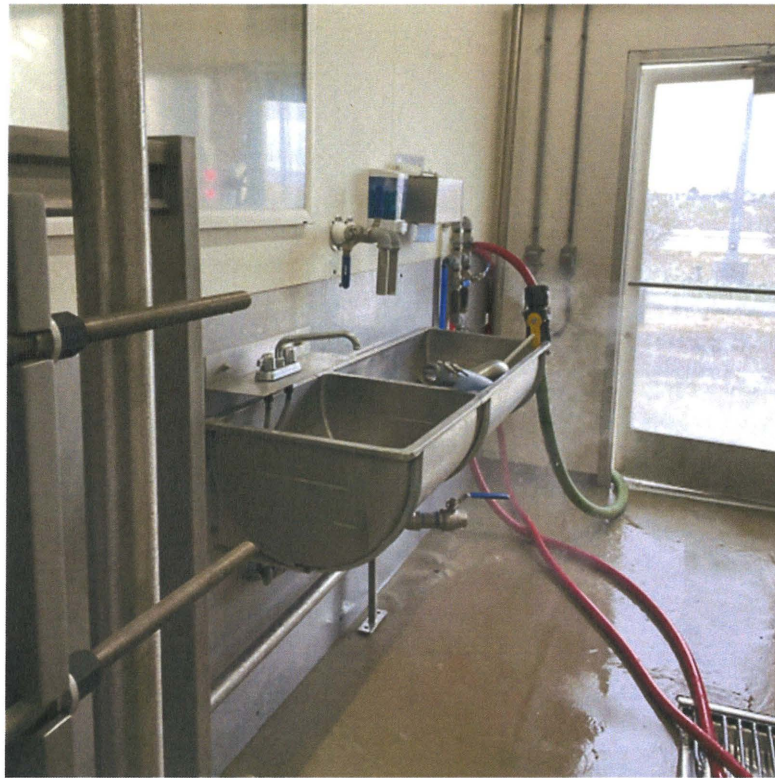
Figure 20 Hand washing sink used intermittently by four employees per day.
