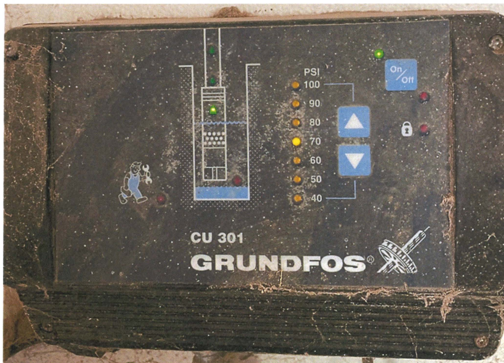
Figure 13 Grundfos CU 301 pressure control panel showing 70 psi for Well 3.
