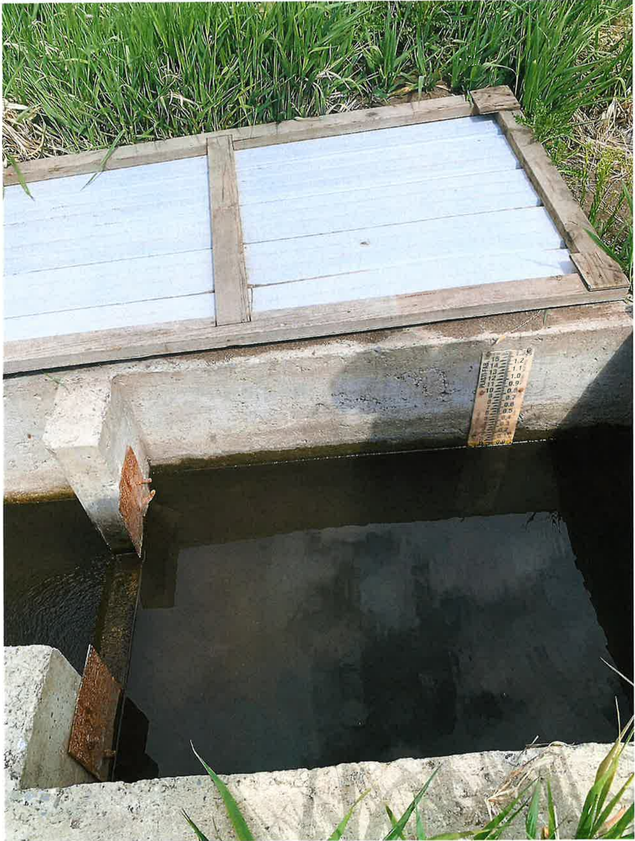
weir at inflow - level zeroed
