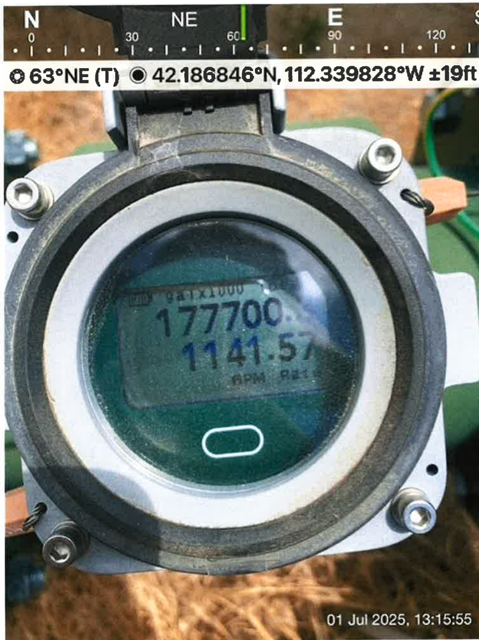
Well SESW Sec 23 Flow Meter
