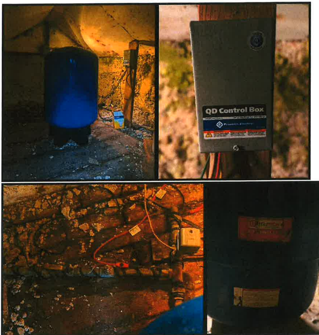
Figure 2. Interior of Spring Collection Pump House – Pressure Tank and Pump Controls, May 16, 2025.
