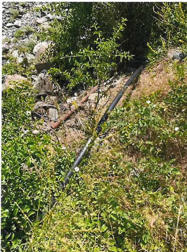
Figure 5: Pipes conveying water from POD to uphill POU
