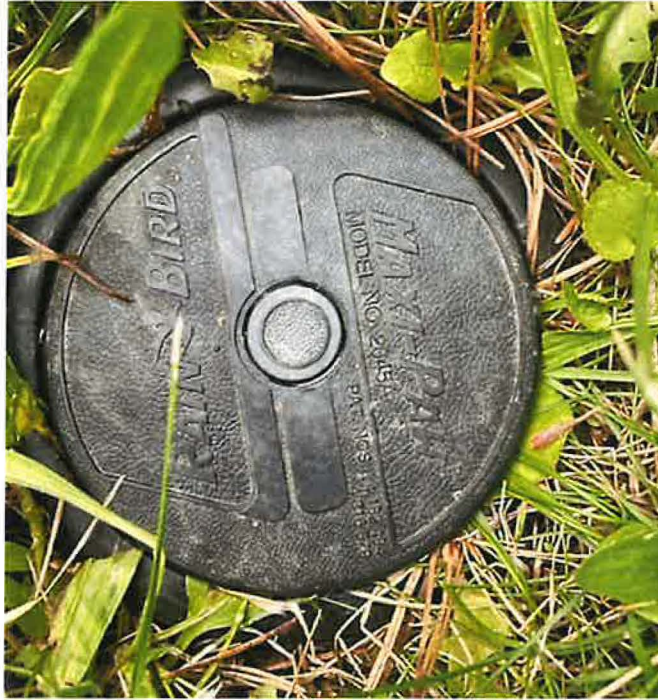
Figure 4: Installed sprinkler irrigation system
