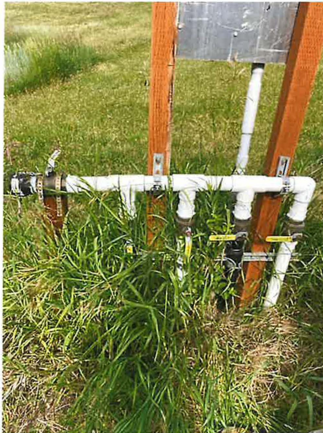
Figure 5: Tee for lines going in, to sprinklers, to orchard, and to fill upper pond
