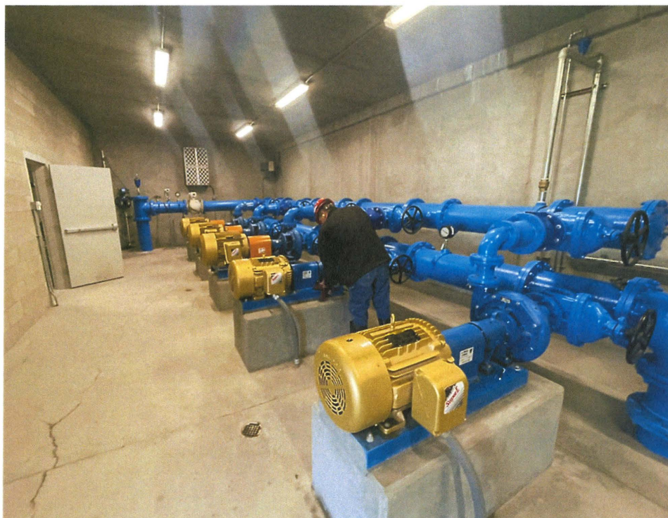
Figure 6 Photo includes the five pump boosters that are associated with Plant Well 1 and system which diverts water to storage tank.
