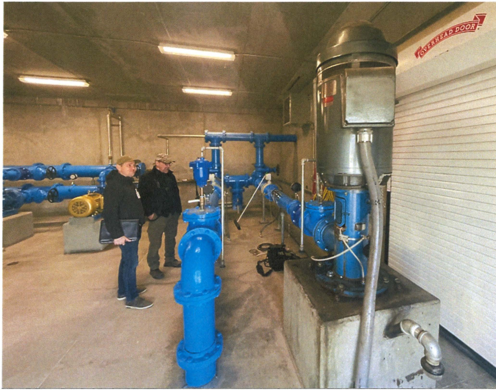
Figure 5 Plant Well 1, D0069003.
