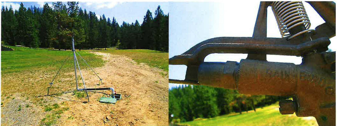
6 Sprinkler Station to 2" Pipe to 1 ½" Galvanized Pipe with 3/8" Rain Bird Sprinkler Head
