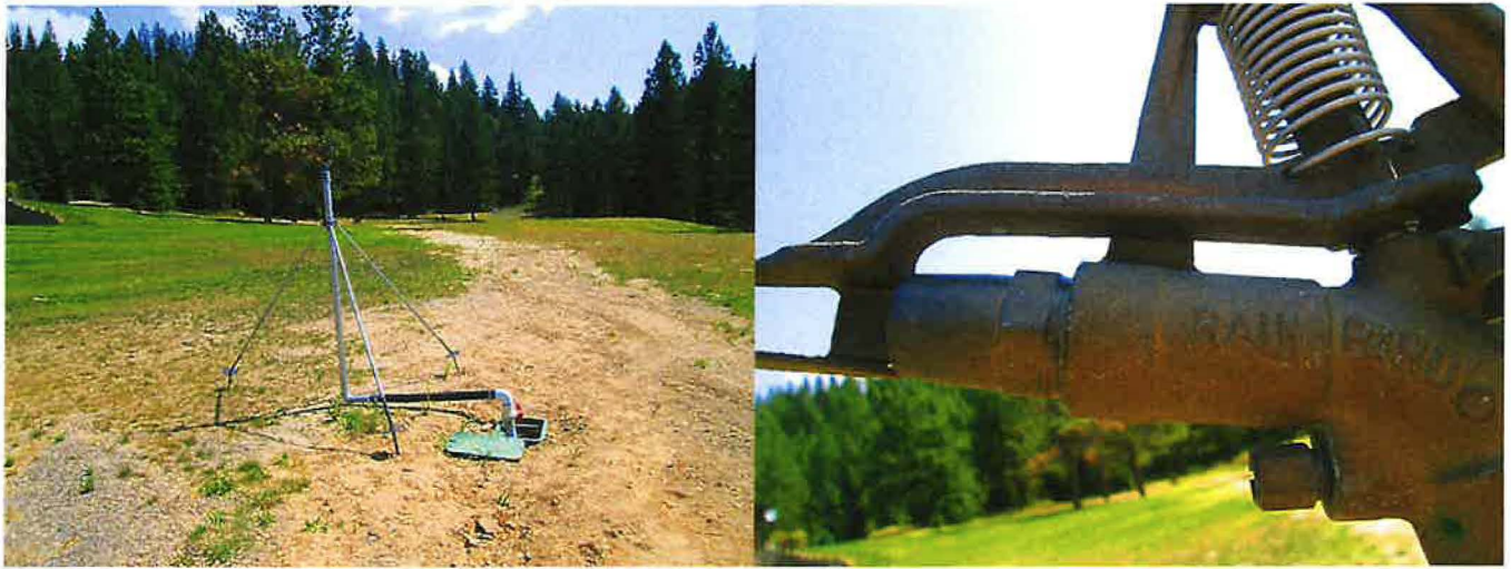
6 Sprinkler Station to 2" Pipe to 1 1/2" Galvanized Pipe with 3/8" Rain Bird Sprinkler Head
