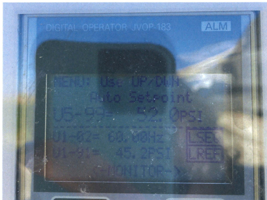
Figure 7 Digital well pump monitor for well D0057945.
