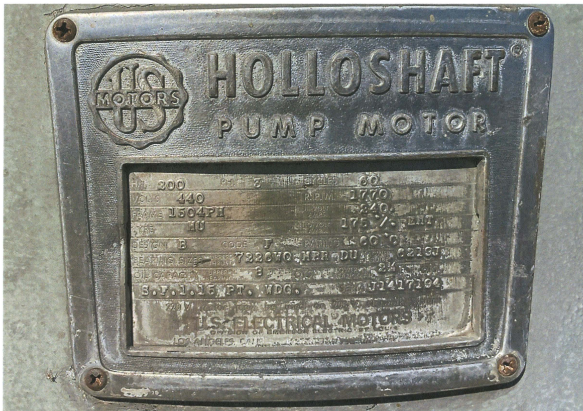
Figure 18 Pump motor specification tag for well 306583.
