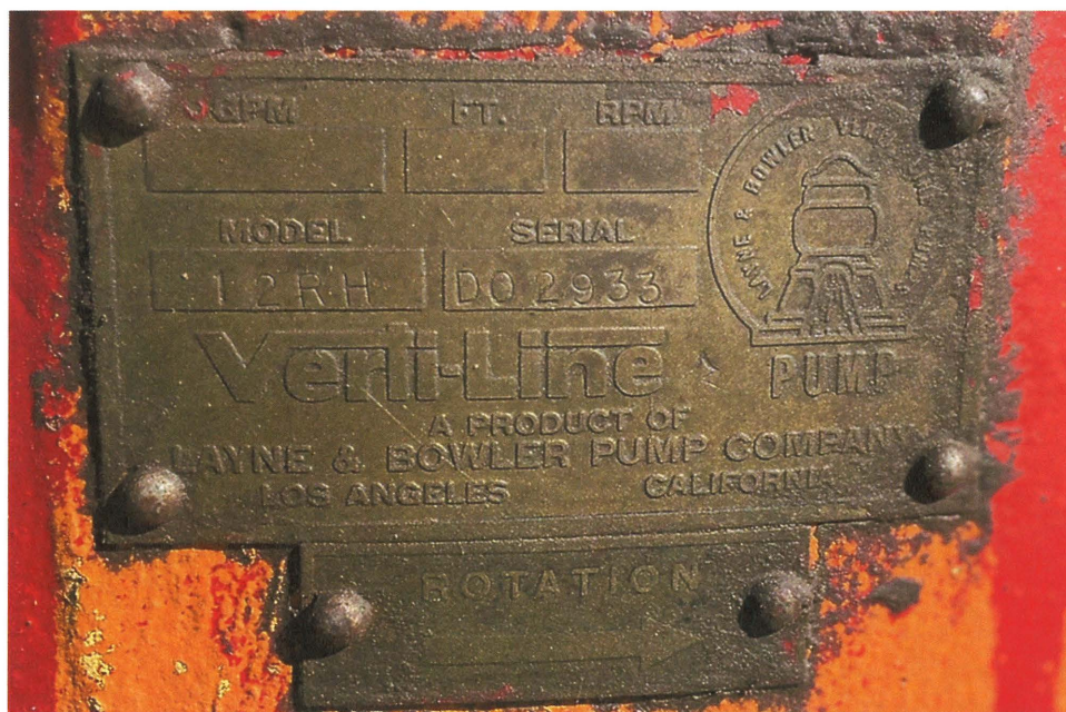
Figure 19 Pump specification tag for well 306583.
