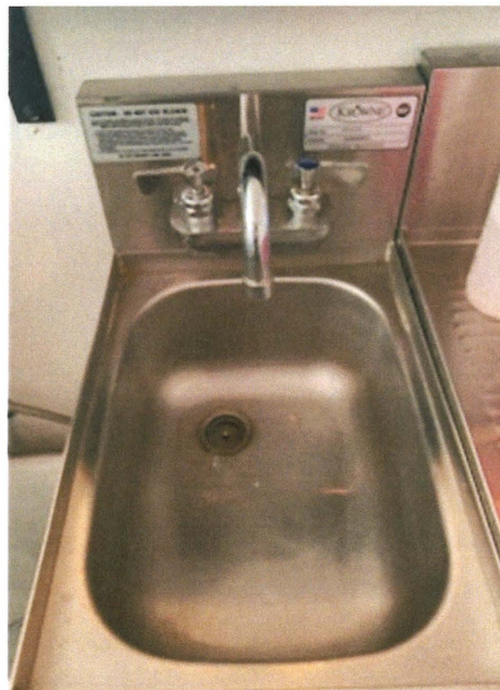
Figure 15 One of two identical bar sinks located in tasting room.
