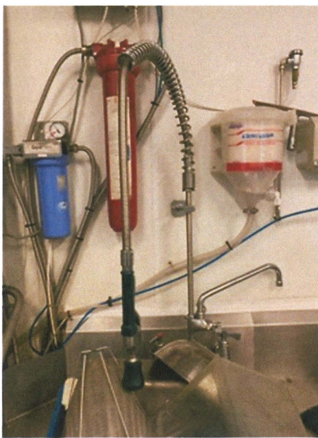
Figure 13 One of two dish sinks used in kitchen.
