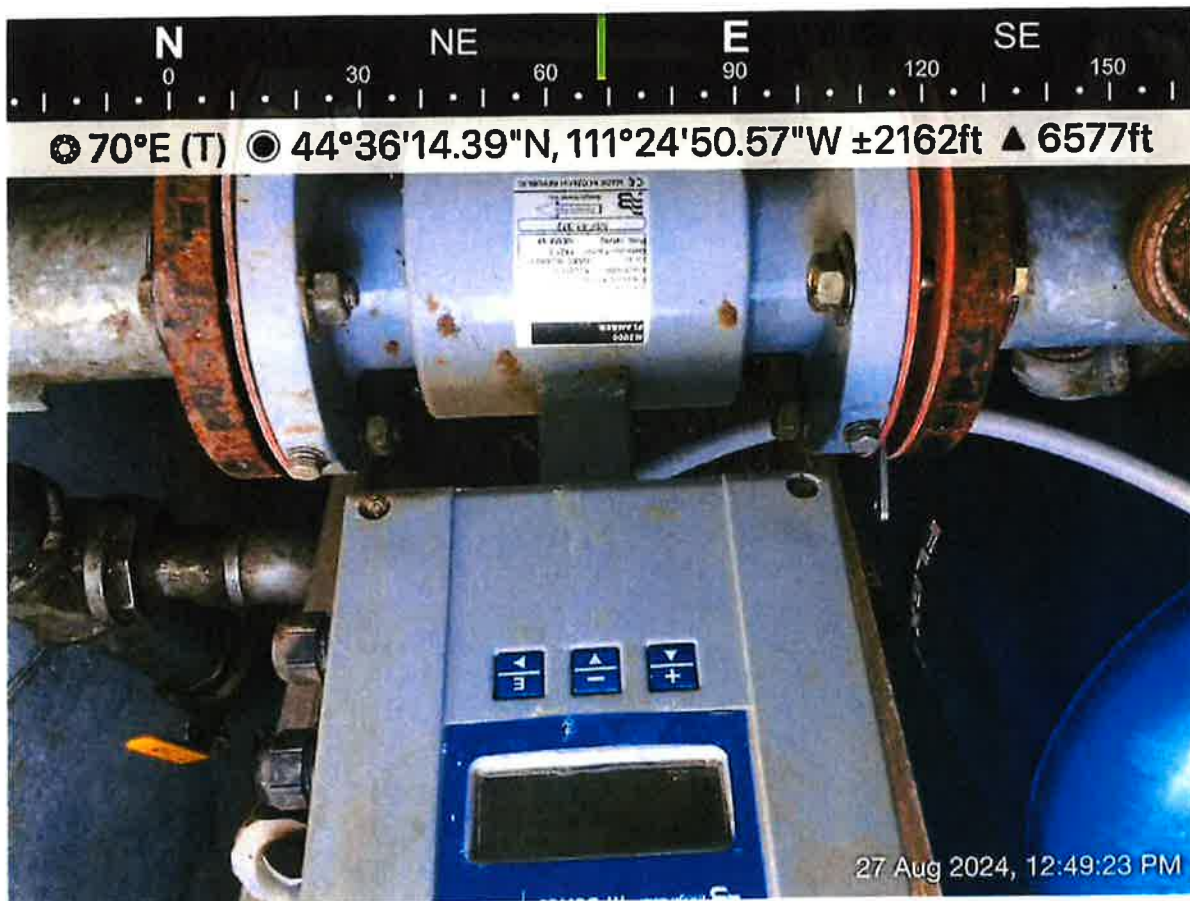
Flowmeter on Well #2
