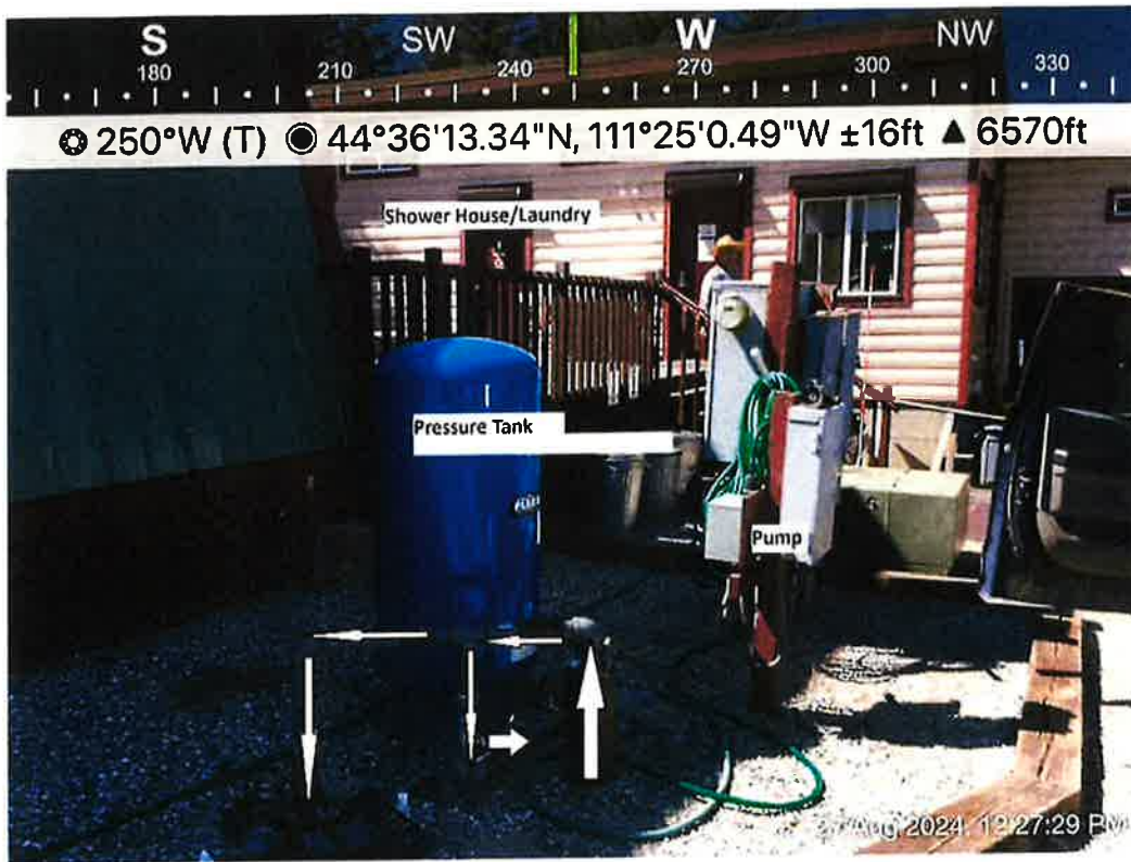
Well #1 D0075936 Well Pump meter
