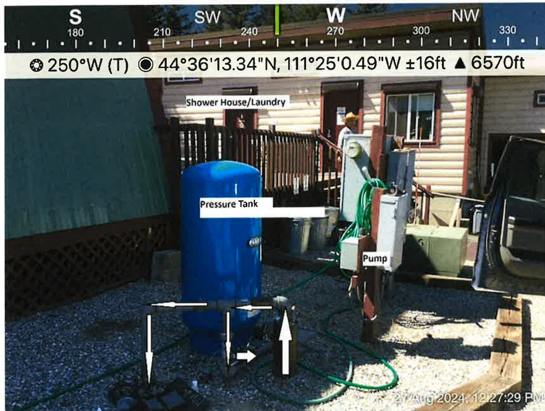
Well #1 D0075936Well Pump meter
