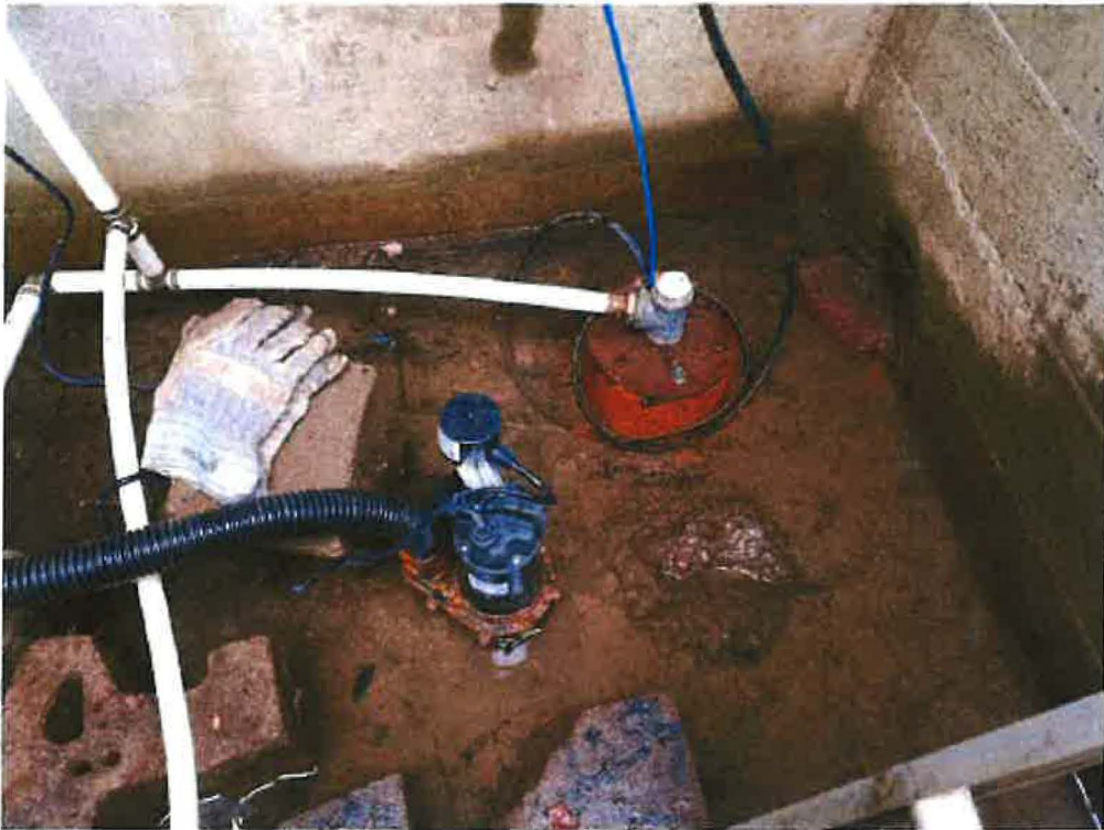
Well Head & Sump Pump
