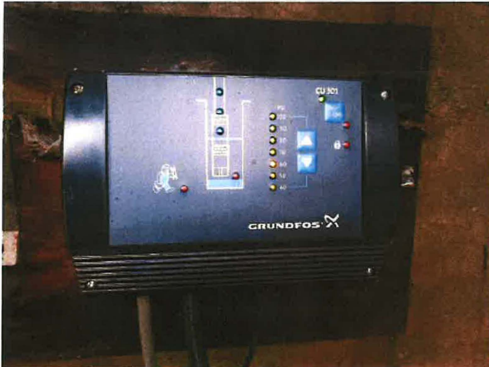
Pump Control Module (2022)
