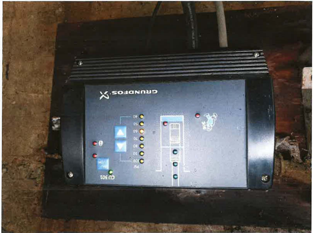
Pump Control Module (2022)
