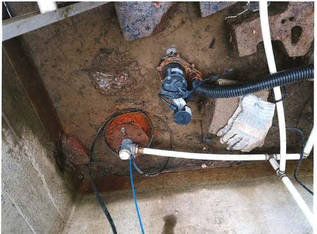
Well Head & Sump Pump
