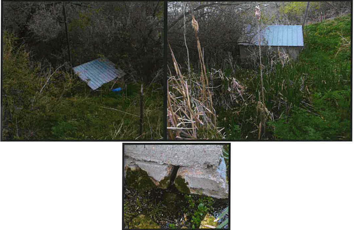
Figure 1. Spring Collection and Pump House, May 16, 2025.
