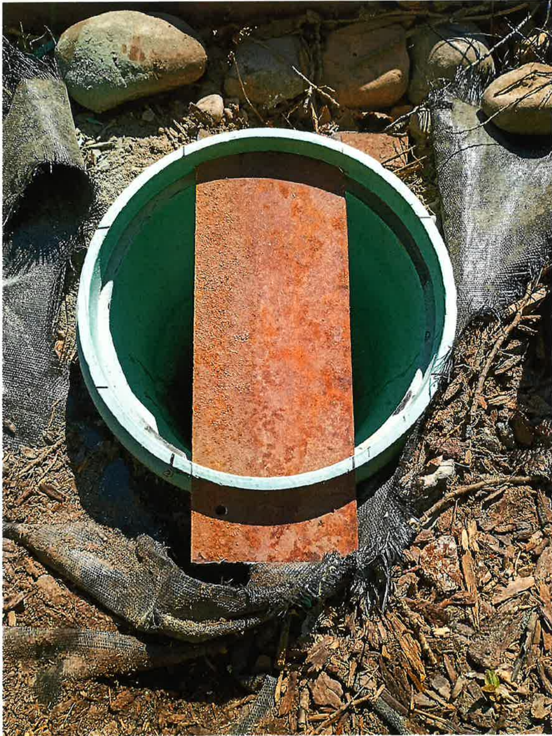
Metal plate with hole to attach a lock to close the diversion
