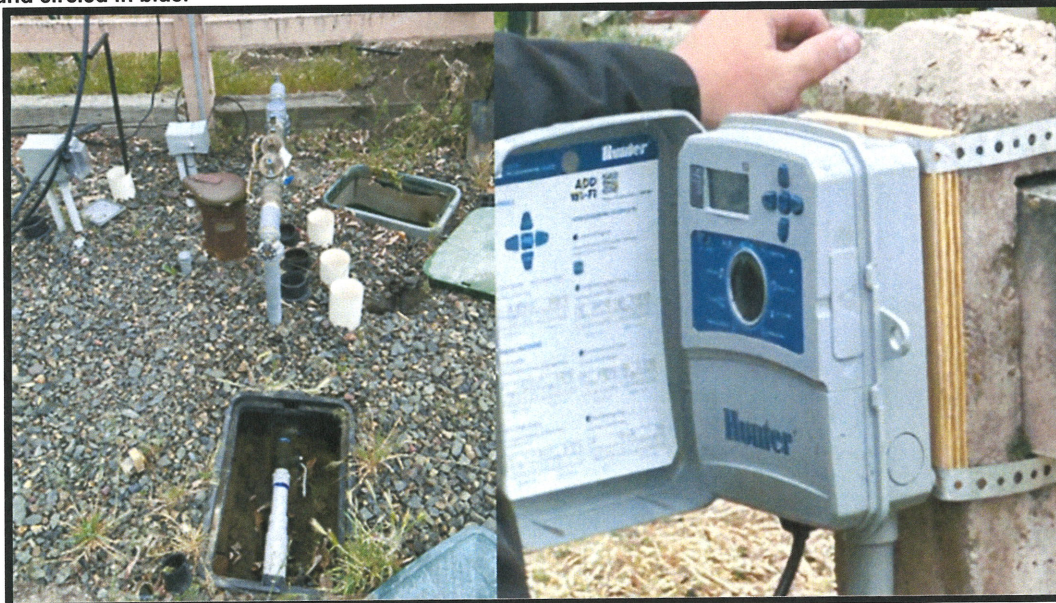
Photos 6 & 7- The check valves and shut off valve on the 1 1/2" PVC main at the old well head (left image). The pasture irrigation timer on the fence post south of the old well head (right image).
