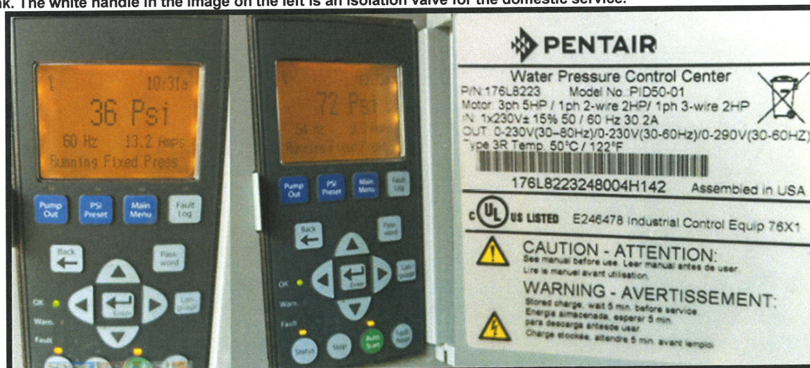
Photos 23, 24, & 25- The pump VFD controller while running the irrigation, domestic, and filling the storage tanks (left image). The domestic service was shut off to allow only water to be pumped up to the water tanks (center image) the upper limit on the controller was set at 70psi. The VFD spec. label (right image).
