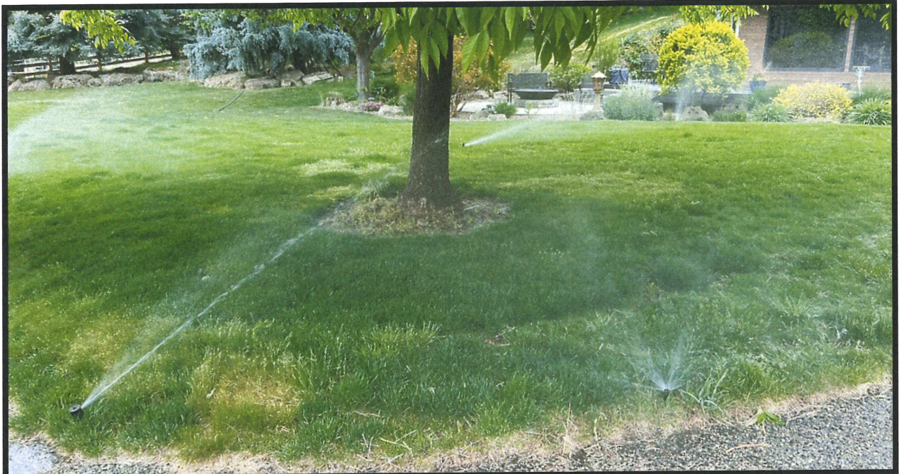
Photo 29- Domestic irrigation system in the southwest corner of the lawn in 2 nd zone with 7 sprinkler heads (Rain Bird 5000).
