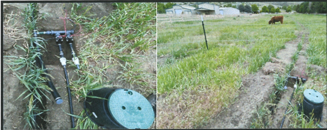
Photos 14 & 15- The control valves for the driplines in the orchard in the western extent of the south pasture areas.
