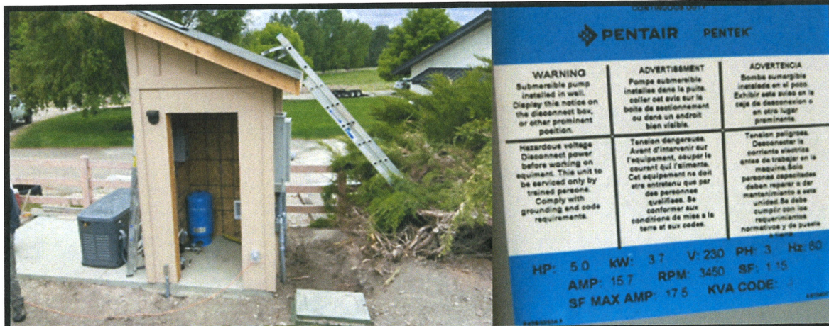
Photos 19 & 20- The "pump house" east of the home has the VFD control, label for the pump, and domestic pressure tank.
