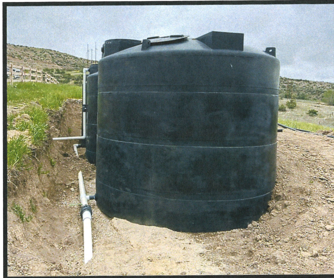
Photo 39- The storage tanks- A 2" PVC fill line enters the top of the center tank. A 3" PVC drainpipe runs between the storage tanks and down the east end of the northwest POU servicing each ditch with a 2" PVC turnout.
