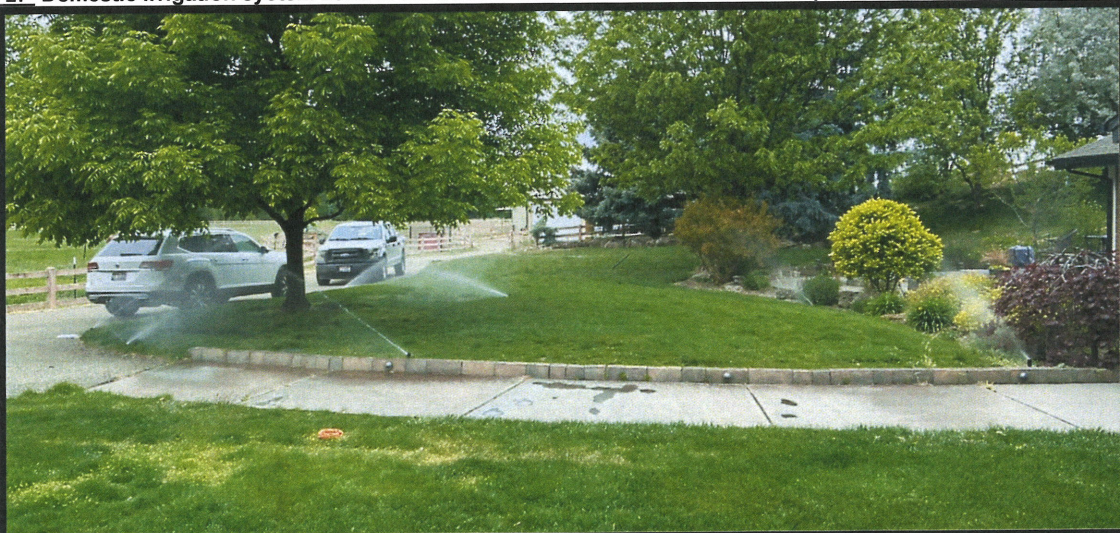
Photo 28- Domestic irrigation system in the southwest corner of the lawn with 7 sprinkler heads (Rain Bird 5000).
