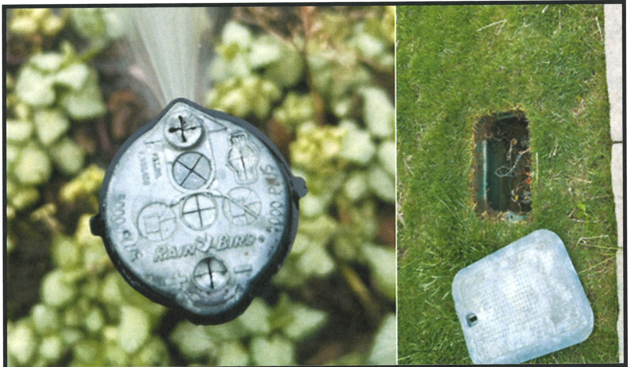
Photo 30- Common domestic irrigation system sprinkler head- Rain Bird 5000 (left image). Control valves in the northwest of the lawn for the western zones (right image).
