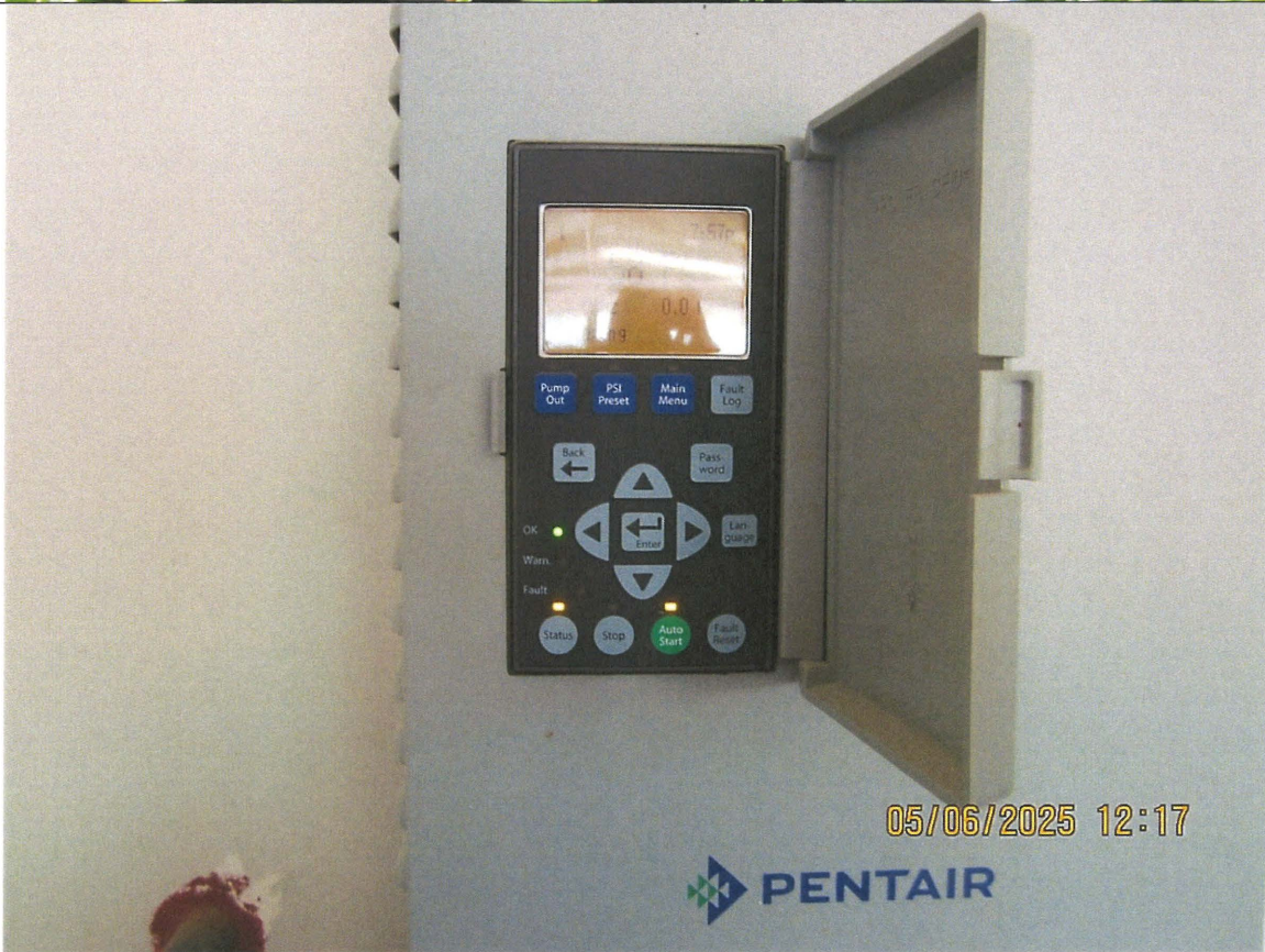
Figure 12. A Pentair Intellidrive, constant pressure controller controls the well pump. The display is reading 58 psi.
