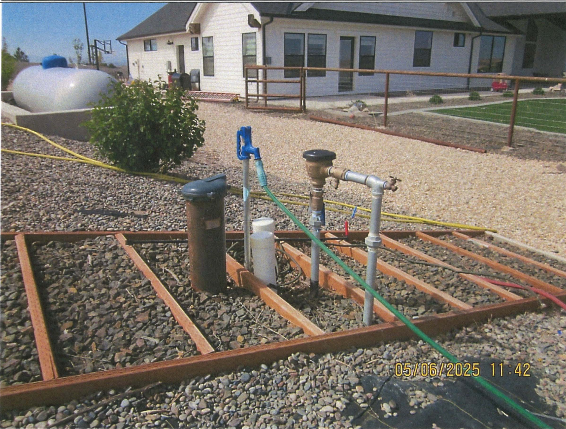
Figure 2. Well head and frost free hydrant.
