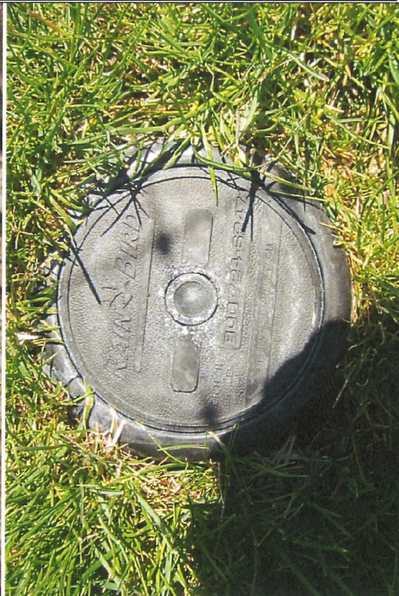
Figure 10. Hunter Pro-Spray PRS30 sprinkler heads were installed in landscaping beds and Rainbirds were installed in lawn areas.
