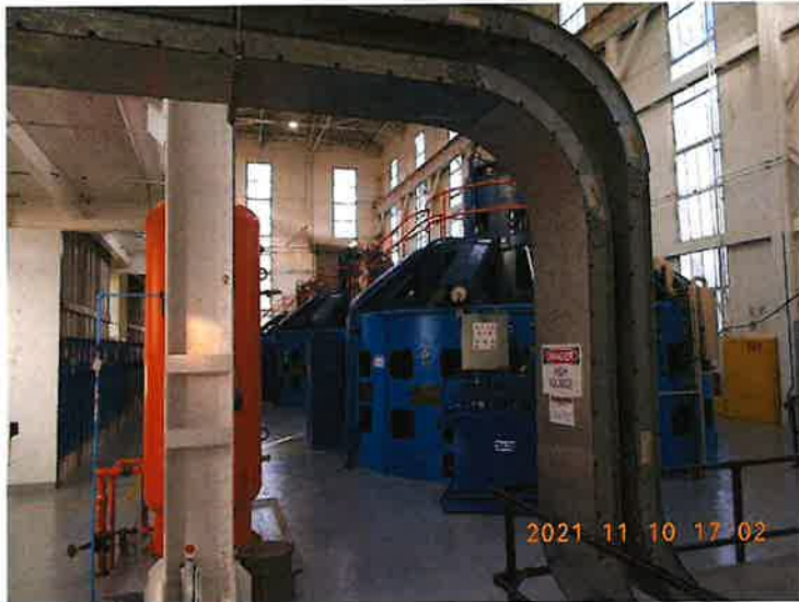
Photo 1. Three turbine/generator units currently in place.
