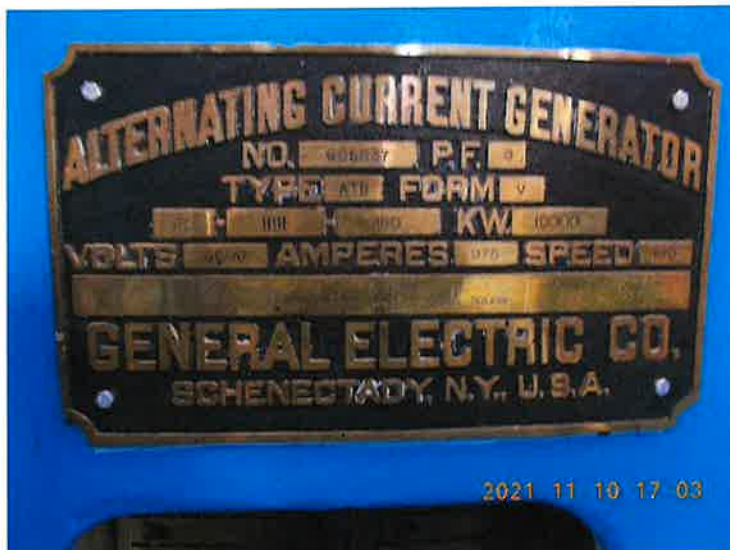
Photo 2. Generator plaque typical of the three units.
