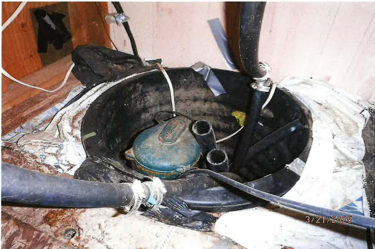
POD – GROUND WATER WELL D0072369 – LOCATED WITHIN UTILITY ROOM STRUCTURE ON LOT 3, BLK 3; BOUNDARY ESTATES SUBDIVISION.
