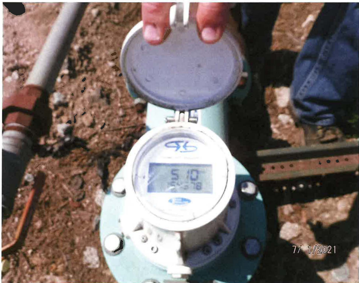
LAGOON DIVERTING WORKS – A VELOCITY STYLE PROPELLER METER, McCROMETER BRAND FLANGED FLOWMETER INSTALLED TO MONITOR 40 HP PUMP. 510 GPM MEASURED AT TIME OF SITE VISIT.
