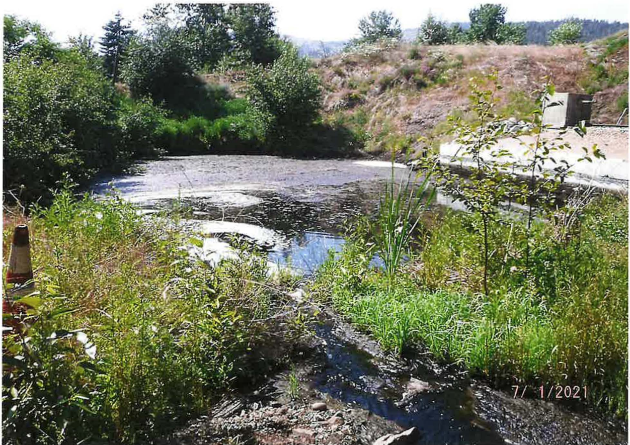
POU – POND #2 (FROG POND) INDUSTRIAL STORAGE & FIRE PROTECTION STORAGE – WATER IS RE-CIRCULATED FOR INDUSTRIAL LOG WATERING FROM THIS POND
