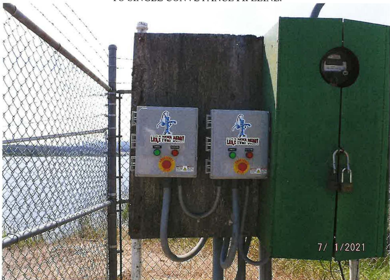
POD – DIVERTING WORKS – 2EA 10 HP FRANKLIN ELECTRIC PUMP MOTORS PAIRED WITH GRUNDFOS PUMP'S PART No. 180STS5 CONTROL PANELS AT LACLEDE BOAT LAUNCH SITE
