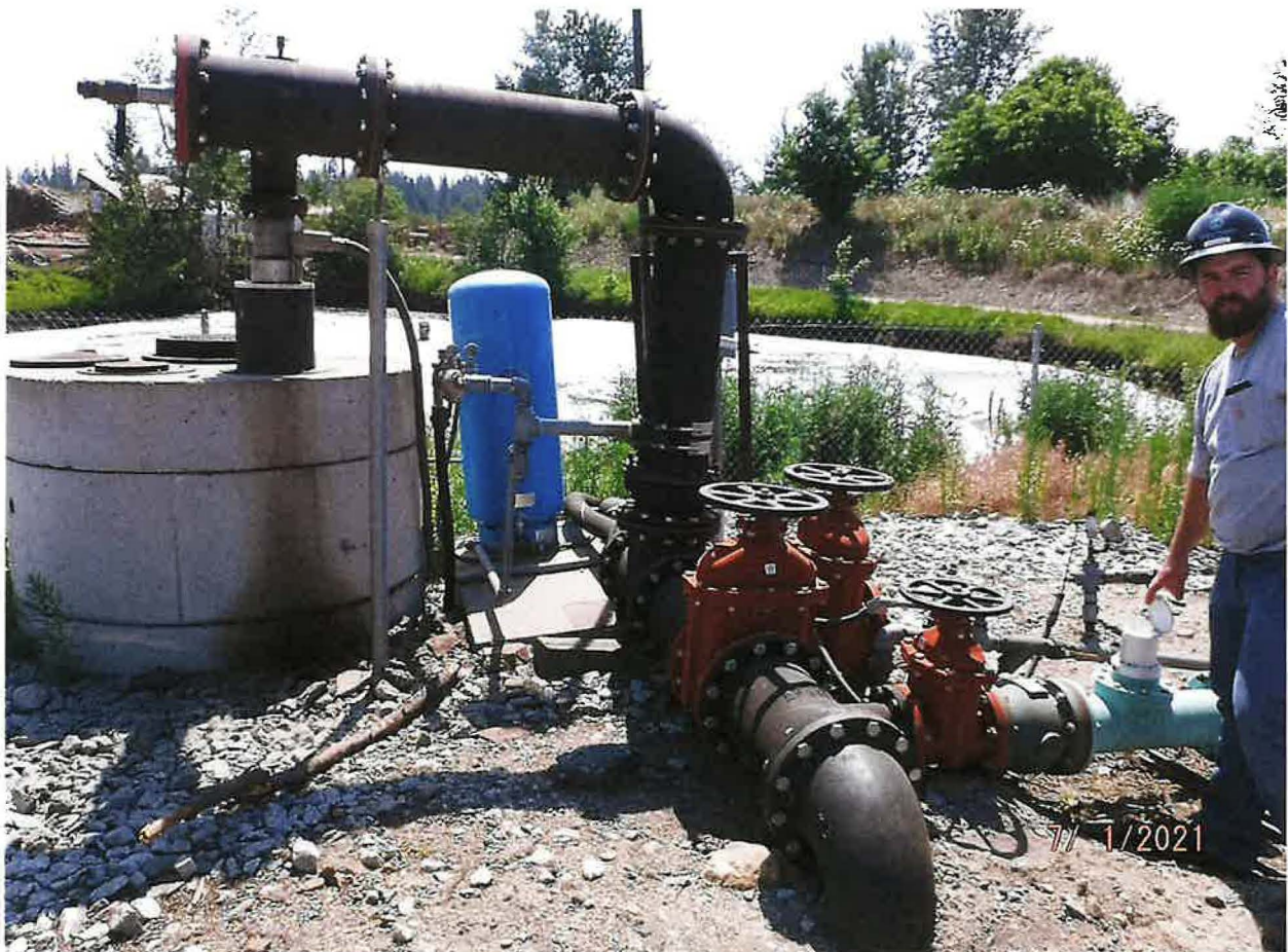
POD – WET WELL FROM LAGOON WITH 40 HP DIVERTING PUMP
