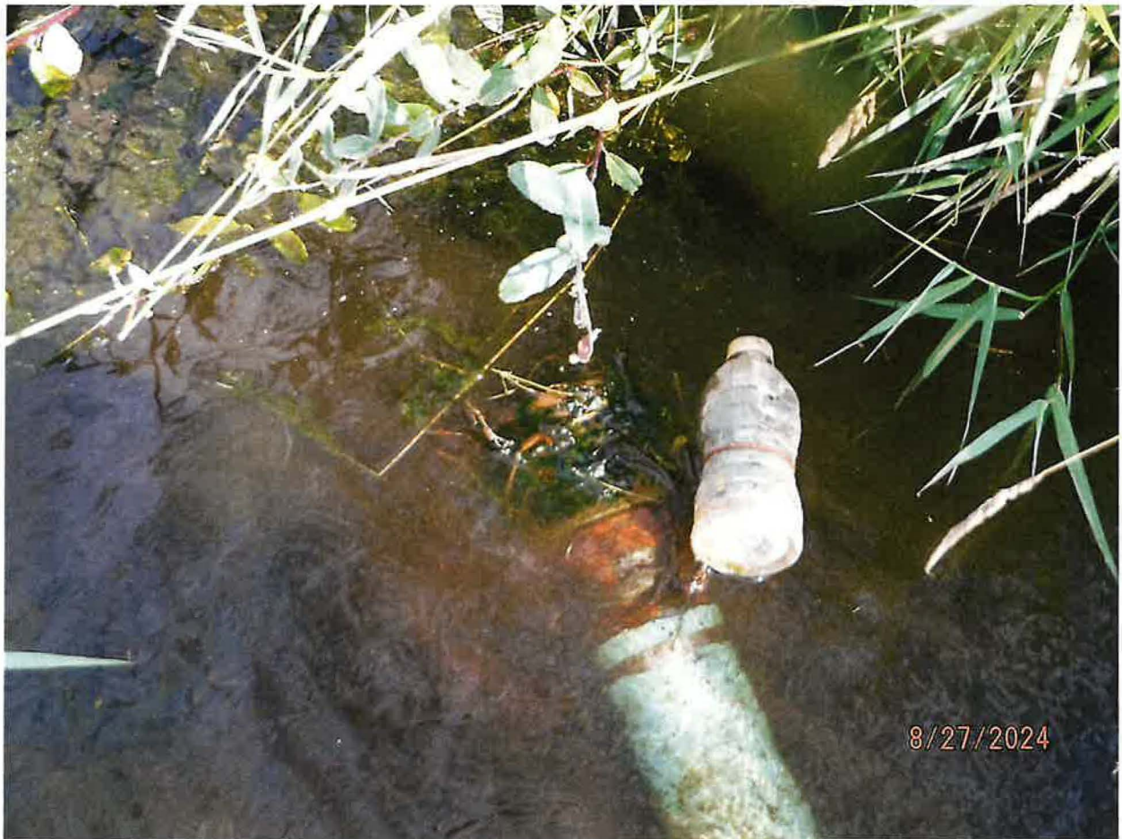
POD – SCREENED 4-INCH INTAKE FLEX PIPE TO GENERATOR MOUNTED TRANSFER PUMP
