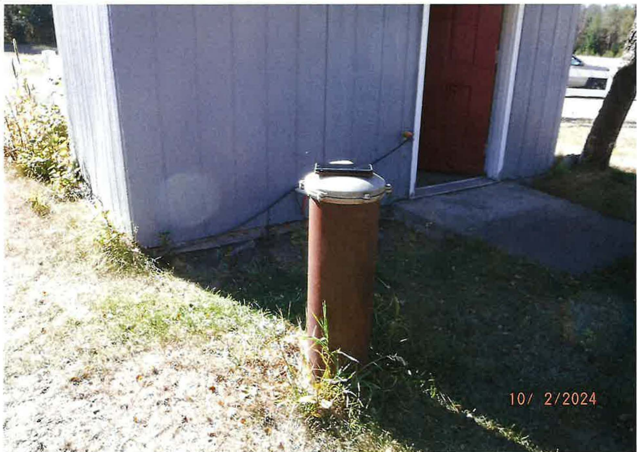
POD – GROUND WATER CASED WELL No. 96-96-N023-000
