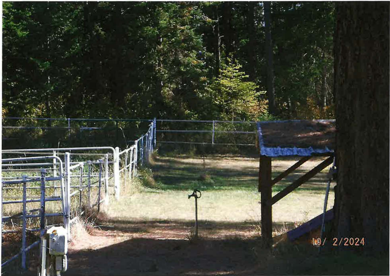
STOCKWATER POU & IRRIGATION POU – ROW OF 8EA FROST FREE HYDRANTS AT INTERVALS WITH HORSE PADDOCKS ON LEFT OF IMAGE & LAWN IRRIGATION ON RIGHT OF IMAGE
