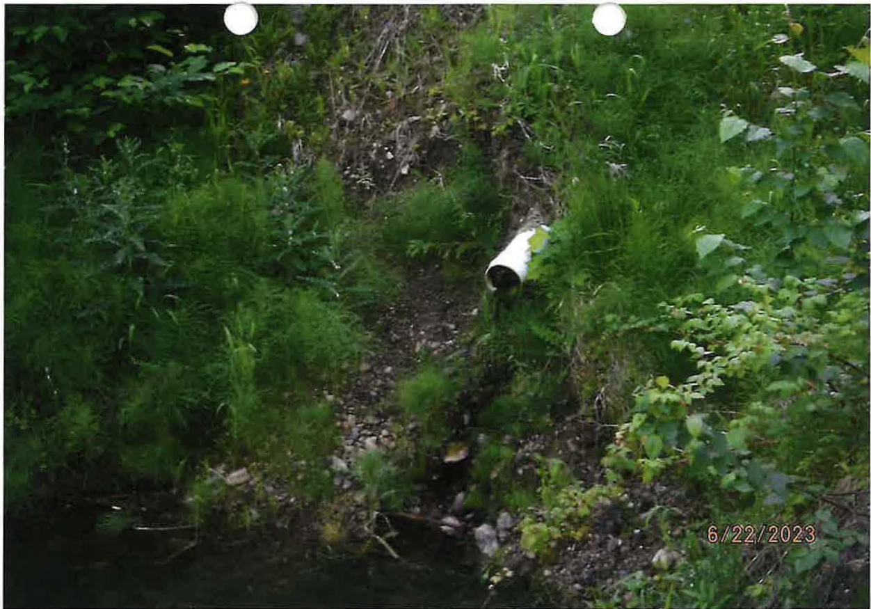
DIVERSION TO STORAGE PVC PIPE FROM STORAGE TANK OVERFLOW TO STORAGE POND; PIPING ROUTES 2-INCH AT STORAGE TANK(S) TO 6-INCH AT INFLOW TO POND
