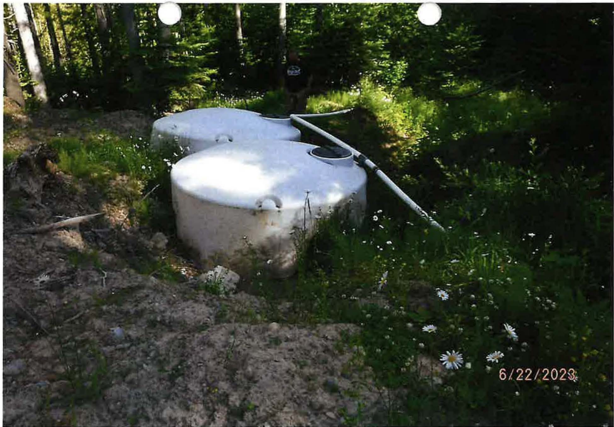
2EA 1,500-GAL ROTOMOLD STORAGE TANKS FILL FROM SPRING PRIOR TO CONVEYING WATER TO STOCKWATER & DOMESTIC USES.
