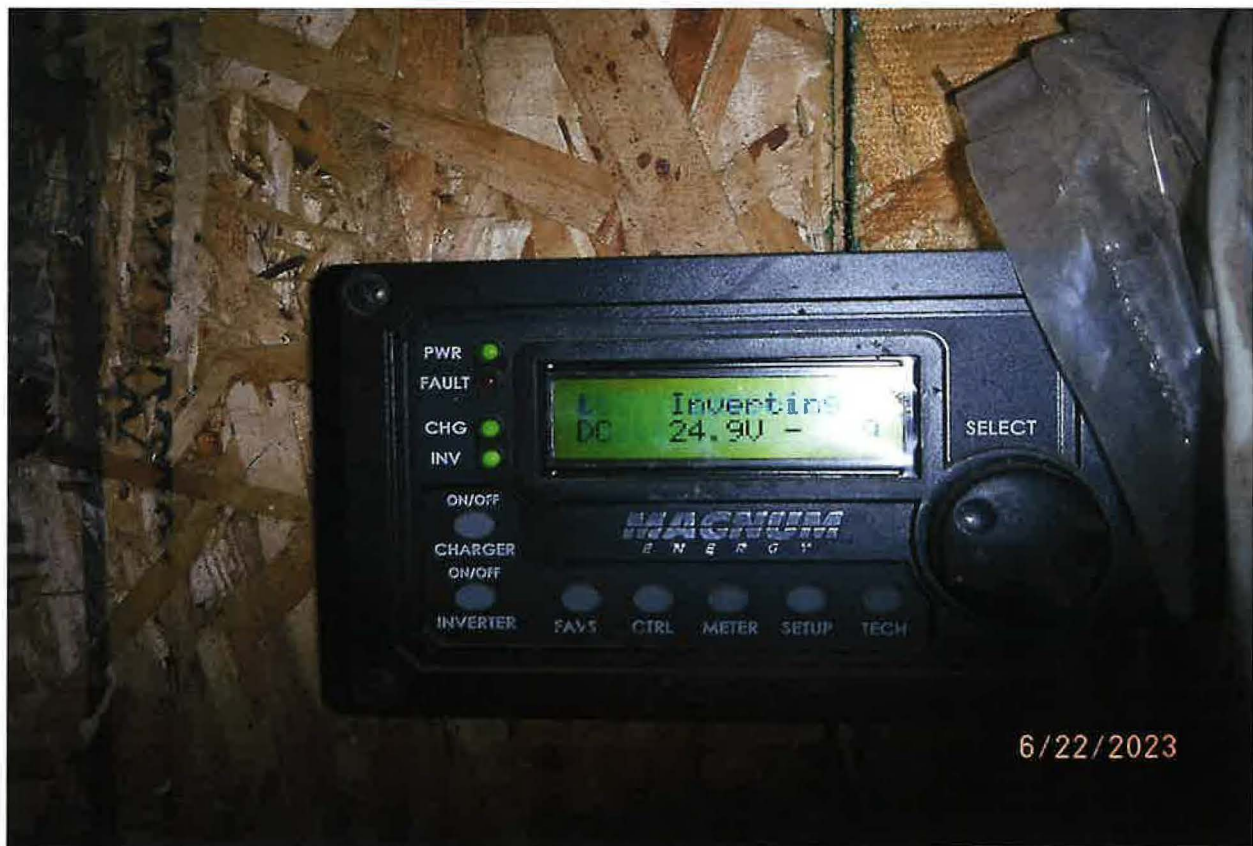
APPLICANT'S MICRO-HYDRO WORKS IN CONCERT WITH A SOLAR POWER SYSTEM – DUAL SYSTEM CONTROL PANEL LOCATED IN THE BARN CO-LOCATED WITH POWER STATION
