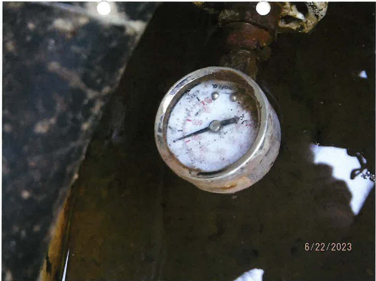
75-80 PSI OPERATING PRESSURE FOR HYDRO POWER SYSTEM
