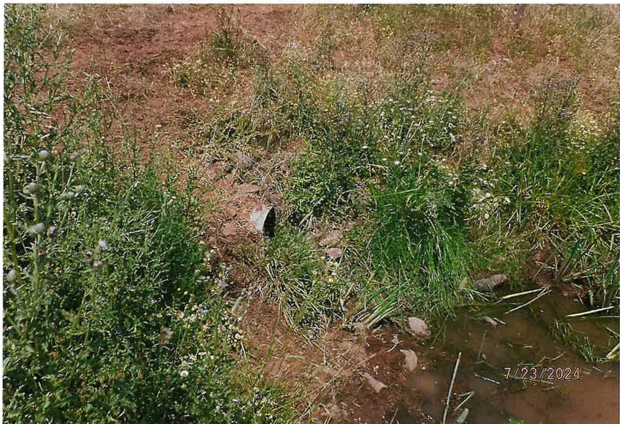
LOWER POND OVERFLOW DISCHARGE PIPE
