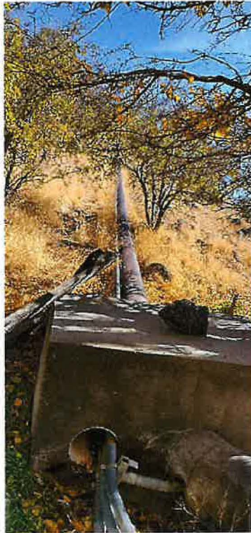
Figure 3: 14" penstock/pipeline to turbines
