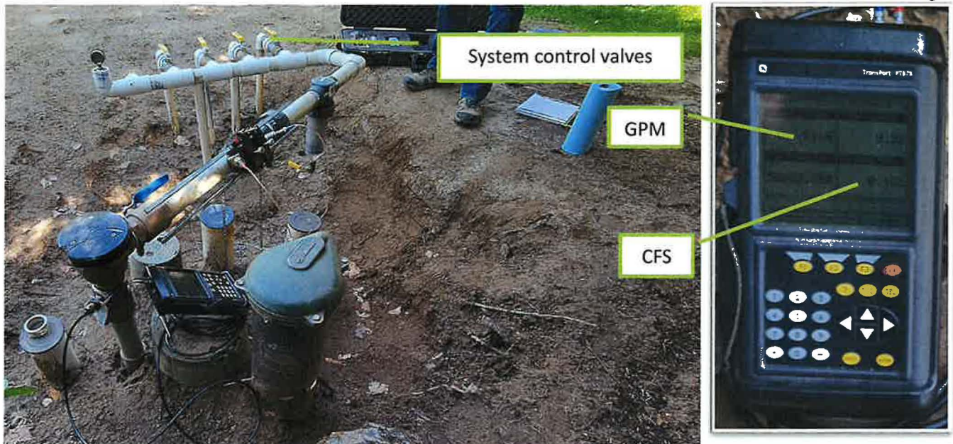
Photo 1: Image of the well head and irrigation system pipelines. Inset image is a picture taken during the measurement showing the maximum flow rate of 81.6 GPM (0.182 CFS).
