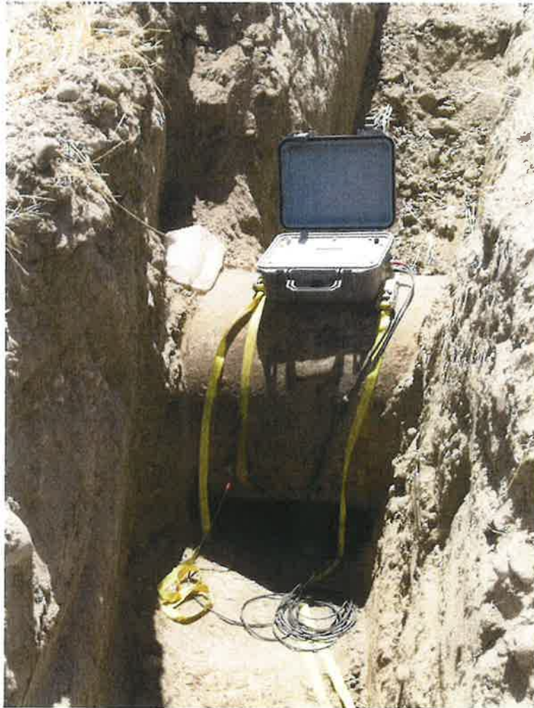
Photo 1. Polysonics Meter installed on Wilson Drain pump discharge pipe.
