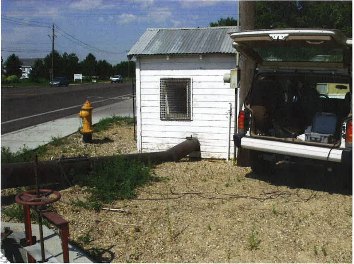
Photo 2. Polysonics meter installed on Post Well discharge pipe.
