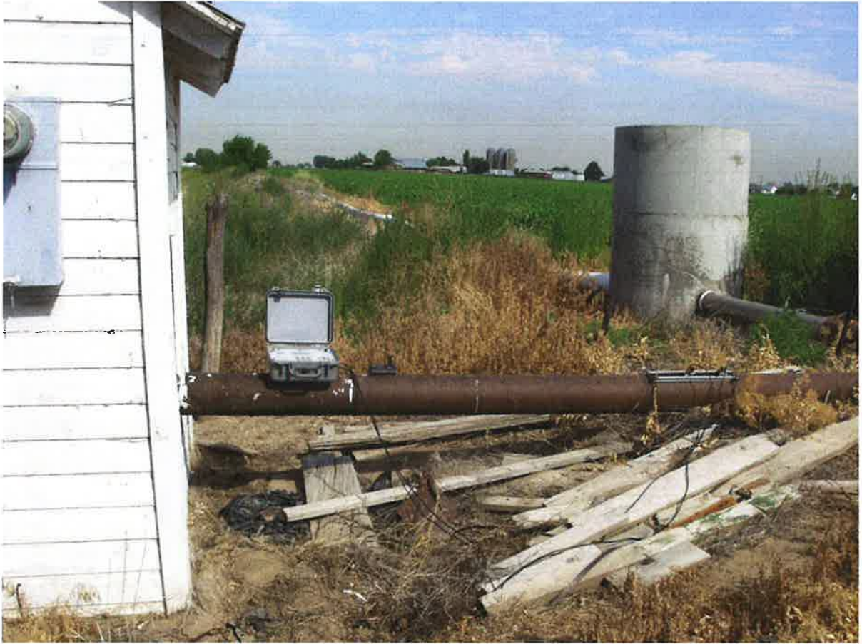
Photo 1. Polysonics Meter installed on Korn Well discharge pipe.
