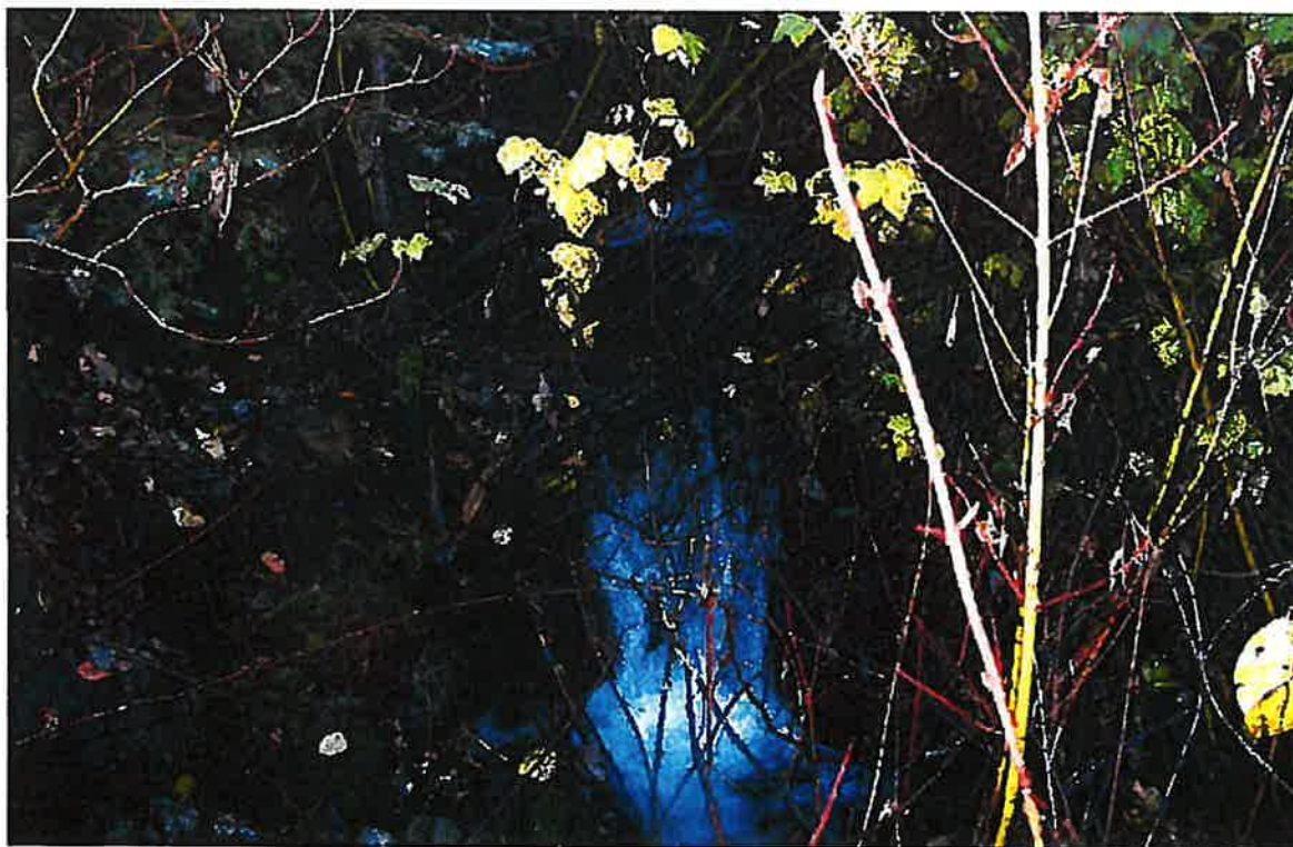
4. Allen ditch culvert outlet at West Mountain Rd. Very overgrown with vegetation.
