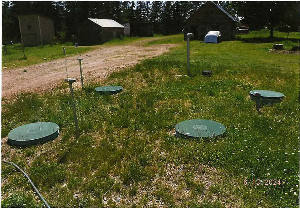
3EA 500-GAL STORAGE CISTERNS & 1EA VAULTED TRANSFER PUMP STATION
