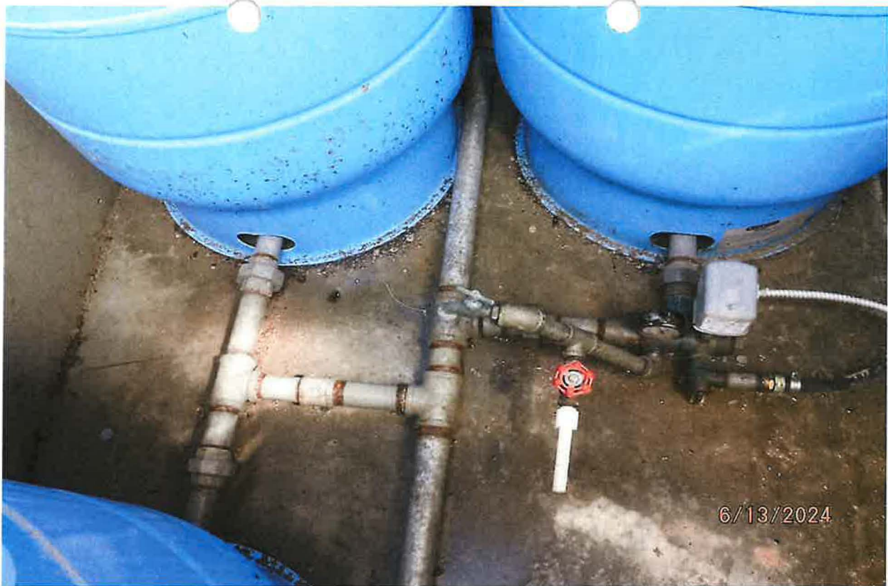
CONVEYANCE SYSTEM INCLUDES 3EA PRESSURE TANKS ASSOCIATED WITH 3EA 500-GAL STORAGE CISTERNS AND 2 HP WATER TRANSFER PUMP FROM CISTERNS
