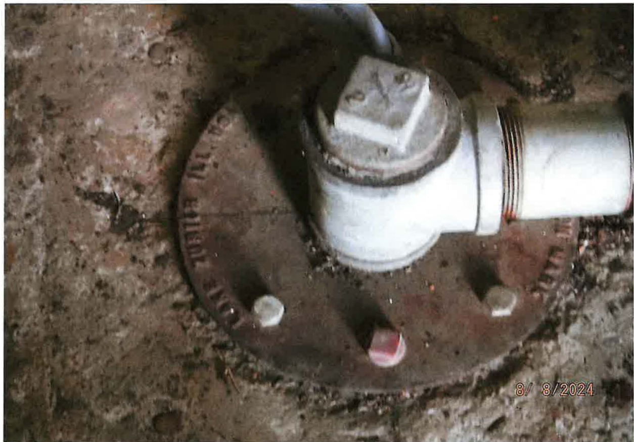
GW WELL – 1960s CASED WELL DRILLED TO 200 FT
