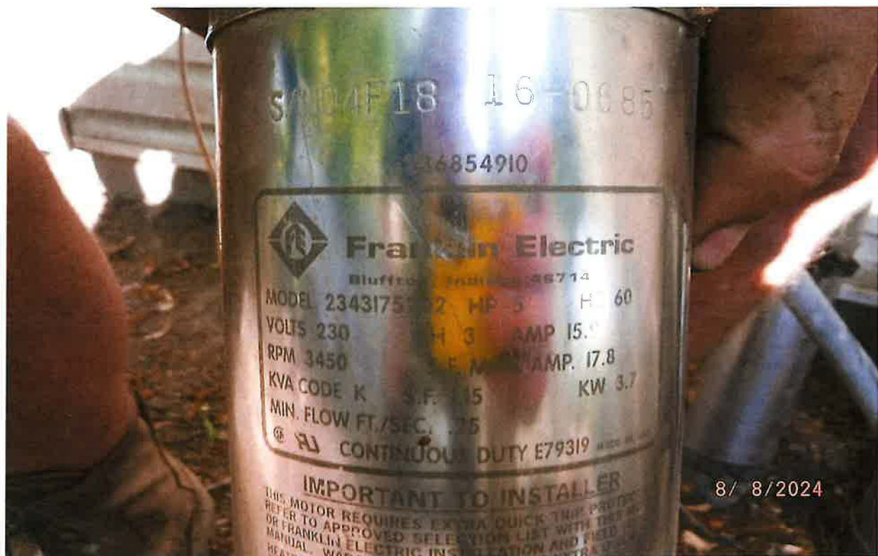
EXAMPLE WELL PUMP END – FRANKLIN ELECTRIC 5 HP, THIS PUMP WAS RECENTLY REPLACED WITH THE SAME MAKE/MODEL AS FOUND AT TIME OF FIELD EXAM
