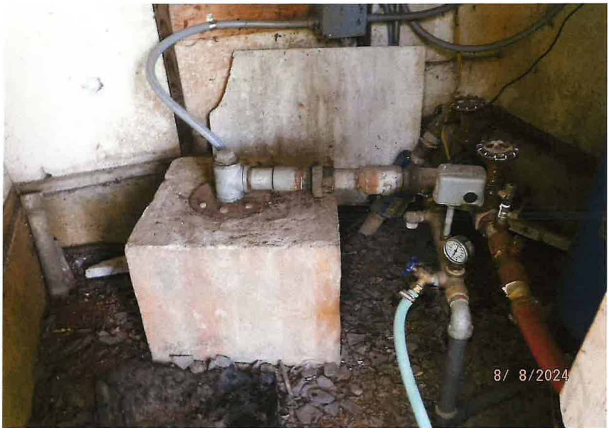
GW WELL AND DIVERTING WORKS HOUSED IN SMALL PUMP STATION
