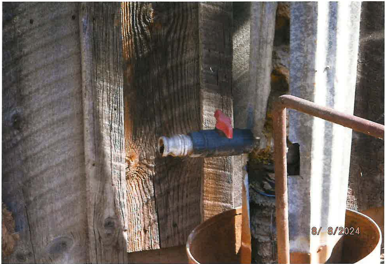
EXAMPLE WATER POINT FROM RISER PIPELINE; SPRAY HOSES CONNECTED FOR INDUSTRIAL CLEANING USES
