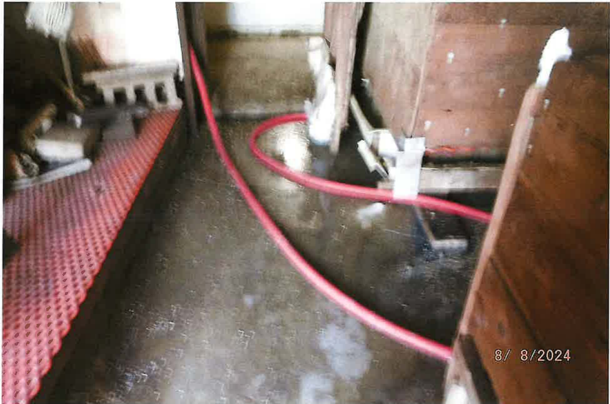
INDUSTRIAL POU – WASH WATER USED REGULARLY TO CLEAN STOCK PENS AND REFUSE CHANNELS – 3-FT X 3-FT DRAIN CHANNELS IN EACH BUILDING
