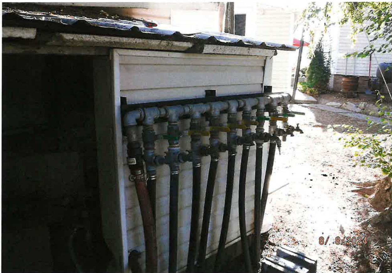
WELL PUMP STATION AND WATER CONVEYANCE DISTRIBUTION MANIFOLD FOR MAIN SERVICE PIPELINES TO WATER USES
