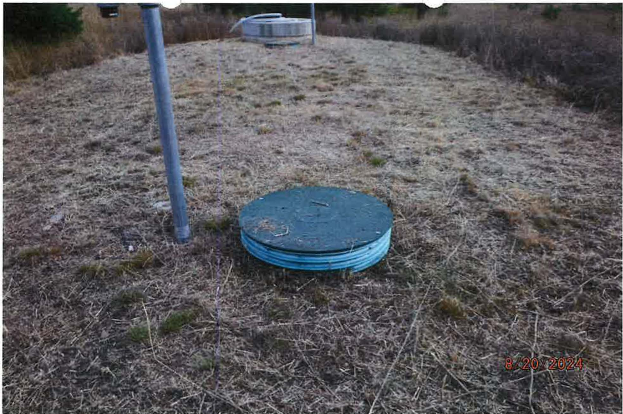
VAULTED STORAGE TANKS BUILT INTO WATER CONVEYANCE SYSTEM
