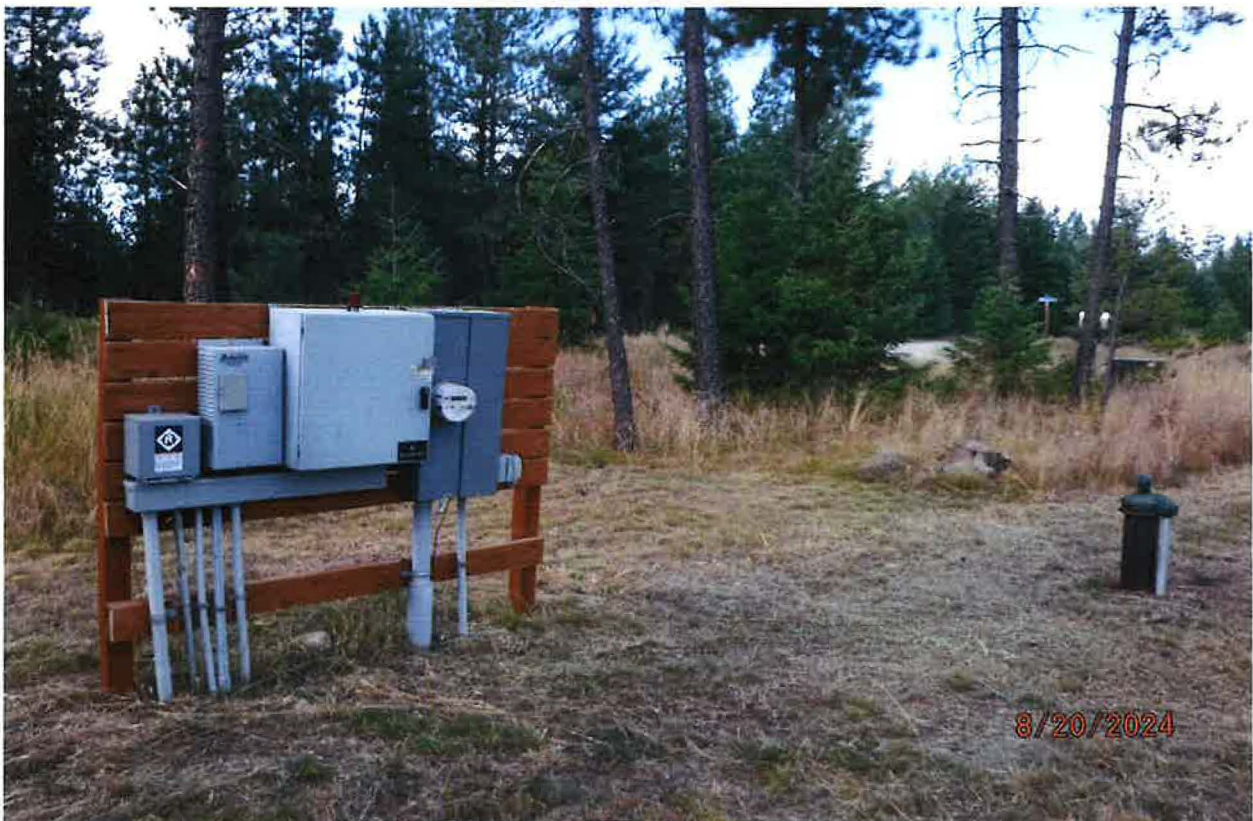
DIVERTING WORKS – WATER SYSTEM CONTROL PANEL(S)
