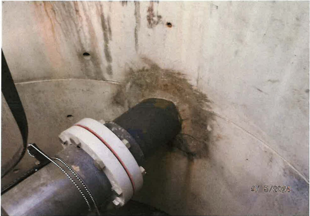
INFLOW FROM WELL TO 30,000-GAL STORAGE RESERVOIR FROM WELL D0079452
