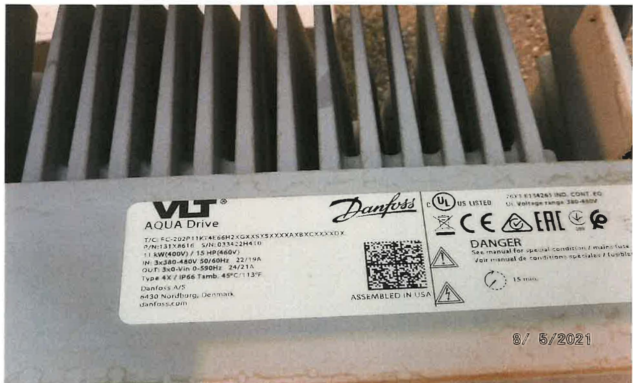
PUMP CONTROL PANEL 15 HP PAIRED WITH 10 HP GOULDS TRANSFER PUMP – FROM RESERVOIR PUMPING TO INDUSTRIAL USES
