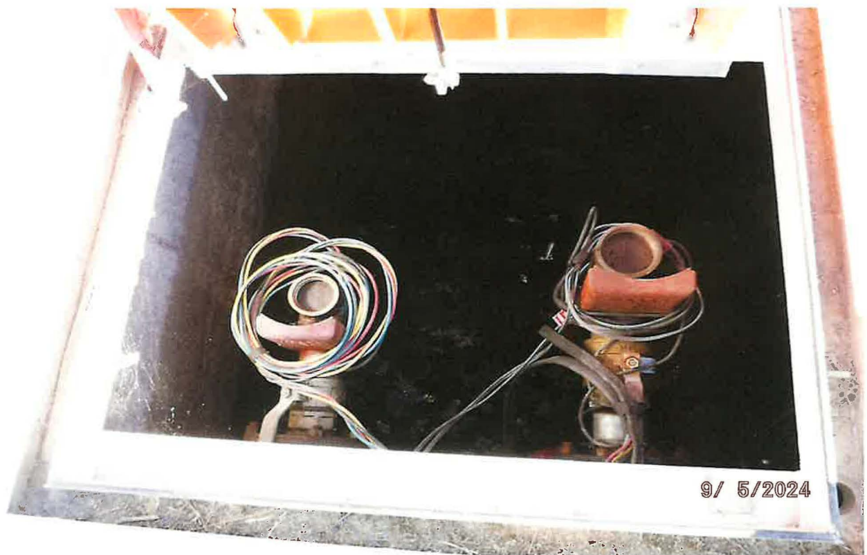
30 HP GOULDS PUMP SET ON PITLESS ADAPTER & 10 HP GOULDS PUMP SET ON PITLESS ADAPTER FROM STORAGE RESERVOIR DISTRIBUTING TO INDUSTRIAL USES
