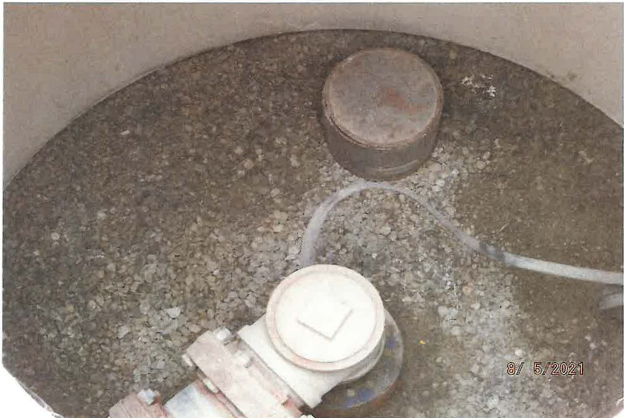
POD – VAULTED GROUNDWATER WELL D0069998 (50 HP GOULDS PUMP IN WELL) & PITLESS ADAPTER
