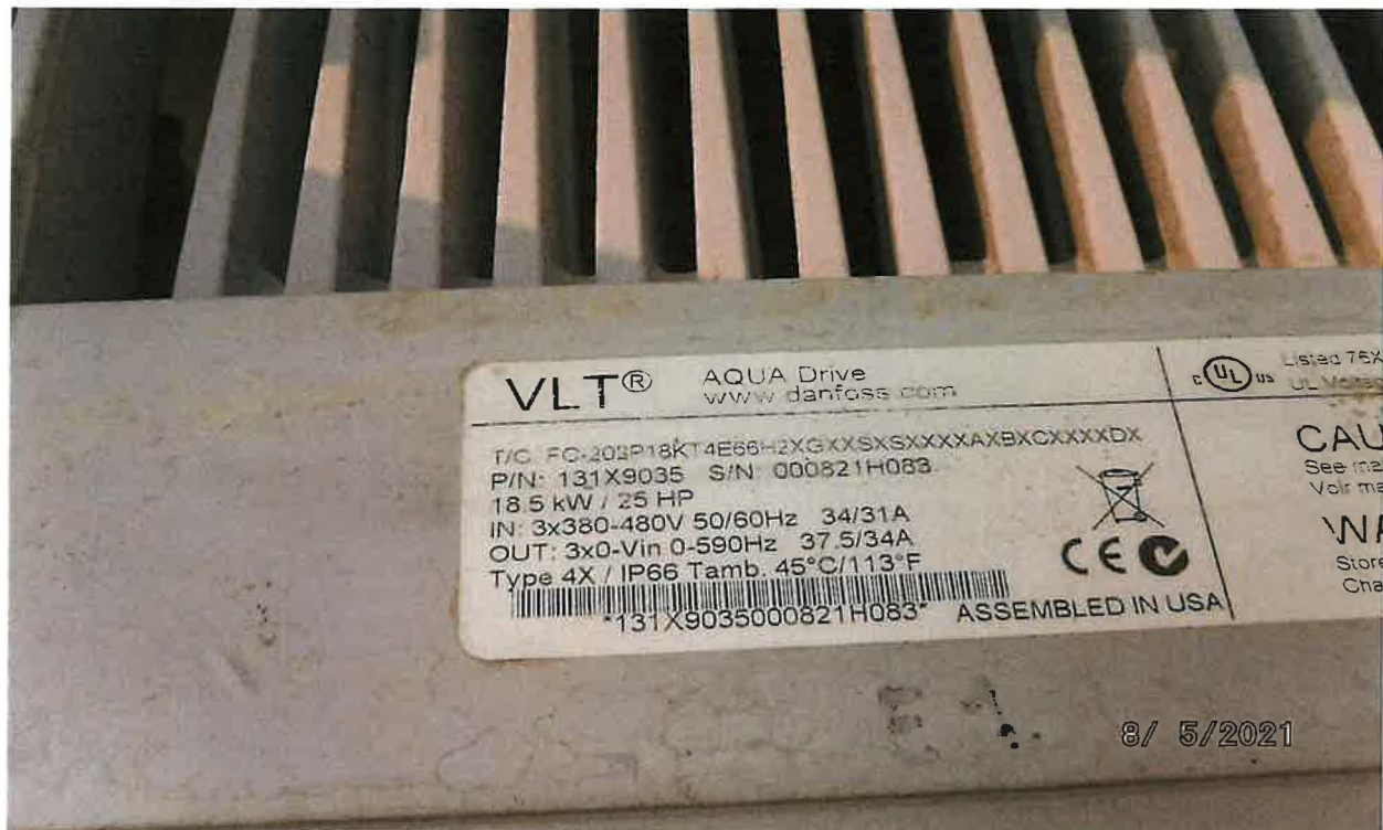
PUMP CONTROL PANEL 25 HP PAIRED WITH 30 HP GOULDS PUMP SET AT LOWER HZ FOR COMPATABILITY AS A DISTRIBUTION PUMP FROM STORAGE RESERVOIR
