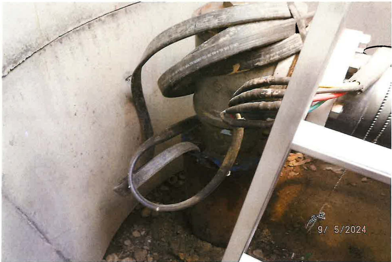
POD – GROUNDWATER WELL D0079452 (50 HP GOULDS PUMP IN WELL) & PITLESS ADAPTER
