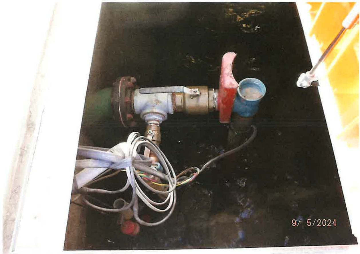
30 HP PITLESS ADAPTER FROM STORAGE RESERVOIR DISTRIBUTING TO INDUSTRIAL USES
