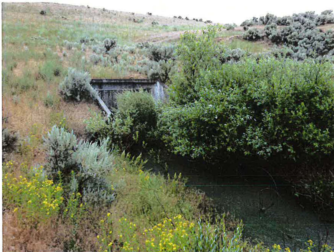
Photo 8: Outlet; note woody vegetation growth next to outlet structure.
