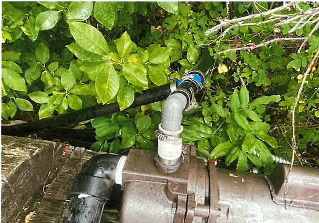
DISCHARGE PIPE REDUCED DOWN TO 1-INCH POLY PIPE
