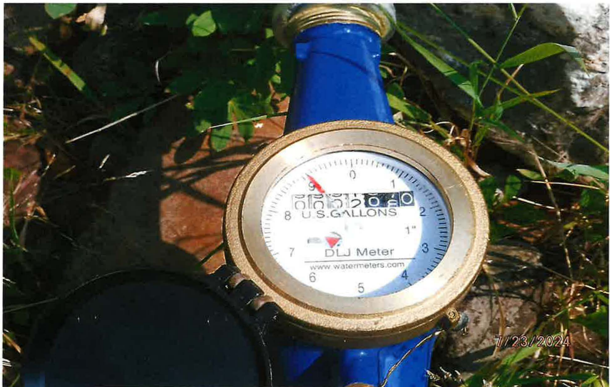
DLJ METER, VELOCITY STYLE FLANGED FLOWMETER INSTALLED INLINE DIRECTLY FROM PUMP
