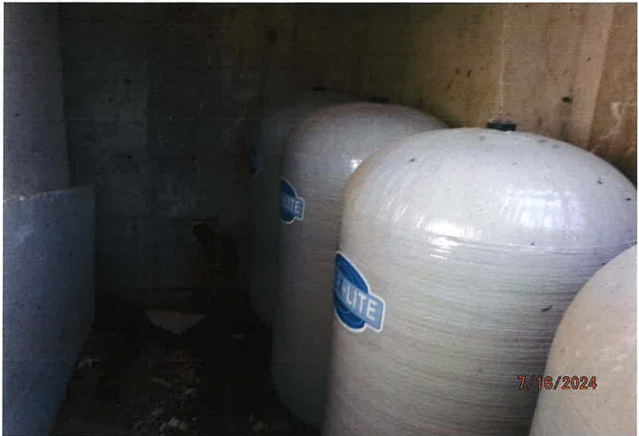
4EA PRESSURE TANKS INSTALLED IN COMMERCIAL CONVEYANCE SYSTEM
