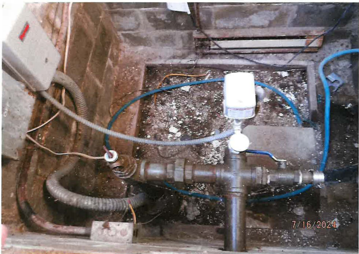
2-INCH METAL PIPE FROM WELL TO PRESSURE TANKS PRIOR TO DISTRIBUTION TO COMMERCIAL USE VIA A BURIED PIPELINE
