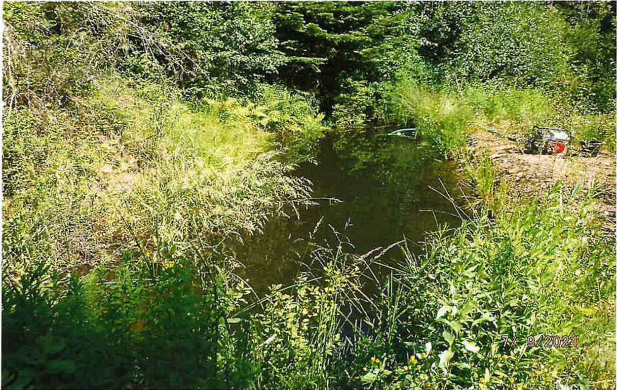
LOWER 24-HR IMPOUNDMENT POOL DEVELOPED OFF-STREAM; 4" PVC PIPE INFLOWS TO POOL FROM CREEK AND 4" PVC PIPE OUTFLOWS BACK TO PIPE. ONCE FULL INFLOW = OUTFLOW.
