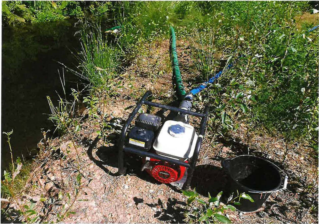
POD – LOWER 24-HR IMPOUNDMENT POOL; GENERATOR FRAME WATER TRANSFER PUMP
